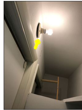
The light fixture is loose.
