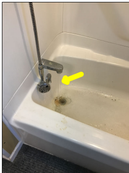
The bathtub faucet leaks while the showerhead is in operation. This is considered a defect. A properly functioning diverter will not allow any water through the bathtub faucet while the showerhead is in operation.
