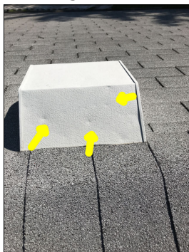
Dents along the roof vents. This is an indication of previous hail damage.
