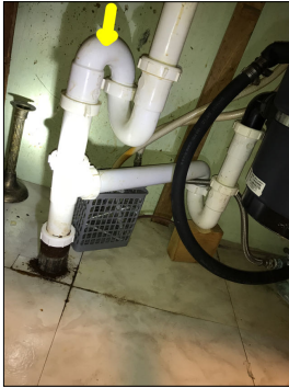
S-trap underneath the sink. S-traps no longer meet modern day plumbing standards. S-traps have the potential to siphon and become dry, thus creating the potential to allow sewer gases into the house. S-traps have the potential to make a knocking/gurgling sound when draining.
