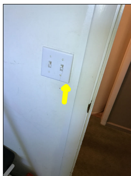
The switches are loose.
