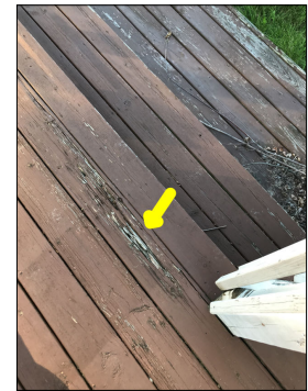
Wood rot damage along the boards.
