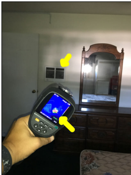
Operable heating elements. The ceiling elements have been disconnected and a wall unit has been installed. This is bedroom 2.
