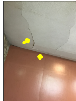
Cracks along the ceiling.
