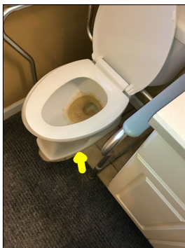
The toilet is loose. The toilet rocks back and forth. A toilet should not have any movement and be fully anchored and secured to the floor.
