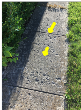
Cracks and deterioration and pitting along the service walks.
