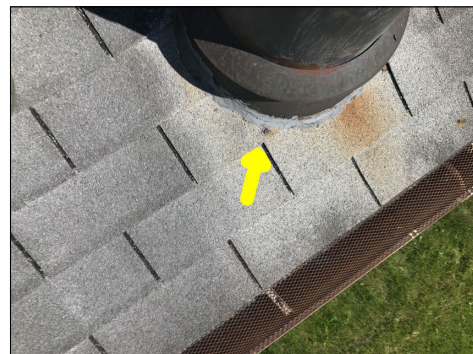
Exposed nailheads/staples. Exposed nailheads/staples are potential leak points.
