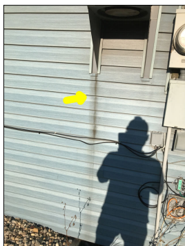
Discoloration along the siding.
