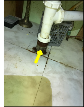
Aged galvanized water lines/pipes. Galvanized pipes no longer meet modern day plumbing standards. Galvanized pipes are prone to corroding from the inside out. Galvanized pipes are towards the end of their life expectancy. Repairs or replacement to galvanized pipes should be anticipated.
