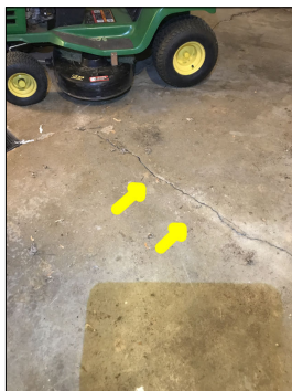
Cracks and deterioration along the floor.
