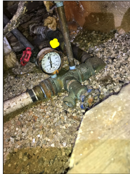
The well pressure was approximately 55 PSI during the inspection.
