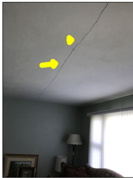
Cracks along the ceiling.
