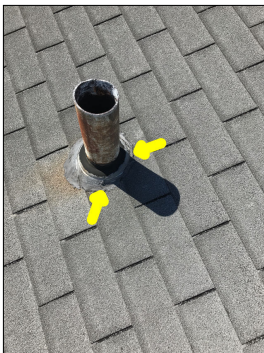
Unconventional application of sealant along the roof. This is considered abnormal and amateur craftsmanship. Amateur craftsmanship is prone to failure and leakage.
