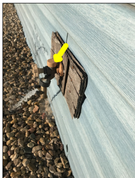
The hose bib is loose. This is considered a defect.
