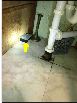
Pest control observed. Wildlife activity can cause property damage.
