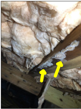
Mold like substance along the floor joists. An active or intermittent water source can cause mold growth and property damage.
