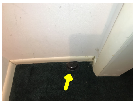
Pest control observed. Wildlife activity can cause property damage.
