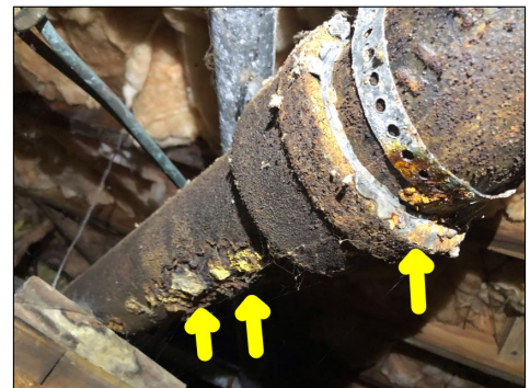
Rust and corrosion along the plumbing pipes.
