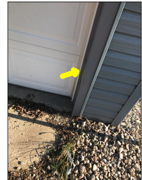
Dents along the siding.
