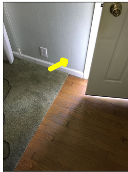
Cracks along the walls.
