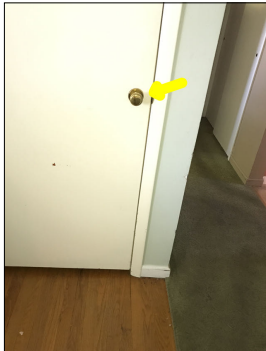
The door does not latch properly.
