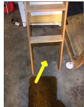
The bottom step is missing from the attic pull down steps.
