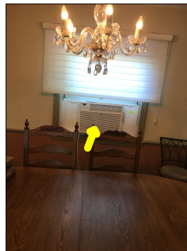
The window was not properly inspected due to the window air conditioning unit inserted into the window. It is beyond the scope of a general home inspection to move personal property. Moving personal property could potentially cause property damage.
