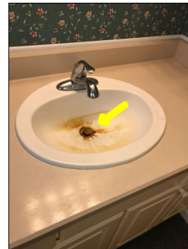
The sink drain is unconventionally noisy when the bathtub is draining. This is considered a defect.
