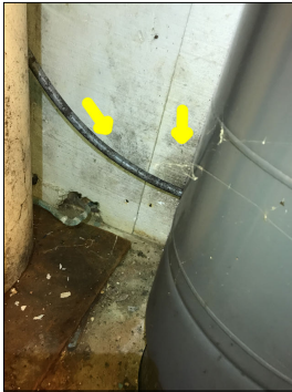
Mold like substance along the wall.
