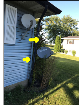
The downspout is loose.
