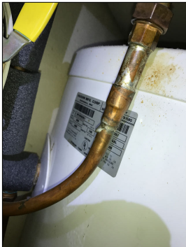
Water heater data plate.
