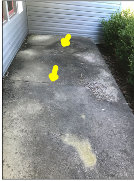
Cracks and deterioration along the porch.
