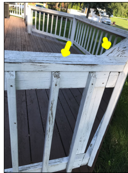
Flaking and peeling along the deck. This is considered a defect.
