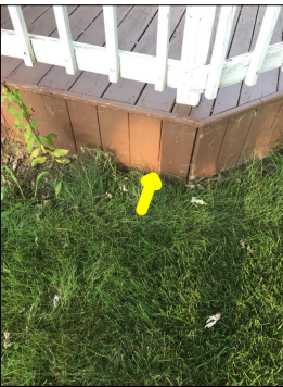
The deck has wood to soil contact. This is not a recommended practice. Water and moisture from the soil/earth can wick up along the deck and the water can be absorbed by the deck. An active or intermittent water source can cause property damage, such as wood rot damage. Also, the wood to soil contact can enable the infestation of wood destroying insects, such as termites or powderpost beetles.
