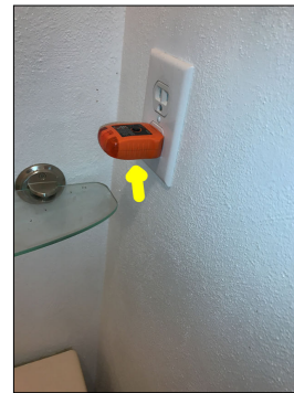
Non GFCI protected receptacles.
