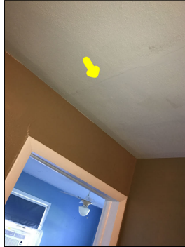
Cracks along the ceiling.
