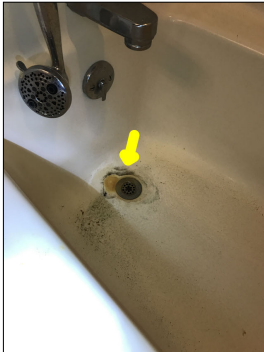
Discoloration along the bathtub. Discoloration can potentially be a mold like substance.
