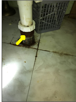
Rust/corrosion along the plumbing pipes.
