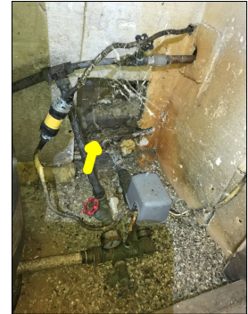
Signs of water damage and moisture observed. An active or intermittent water source can cause property damage and mold growth.
