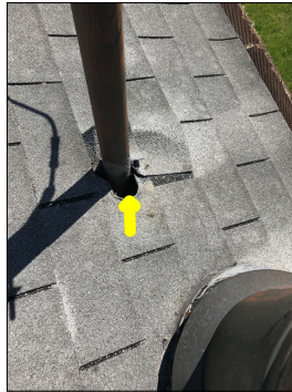
Hole along the roof.
