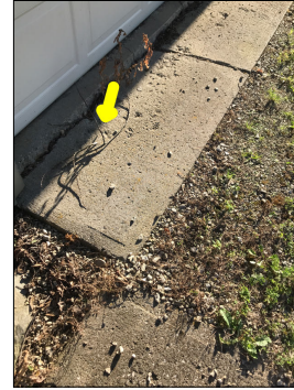
The driveway slopes towards the house. This can cause water to flow towards the house, thus potentially causing water intrusion into the house/garage and potential foundation problems due to excessive hydrostatic pressure.
