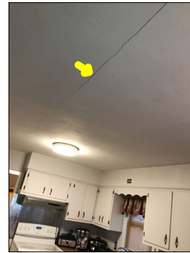
Cracks along the ceiling.
