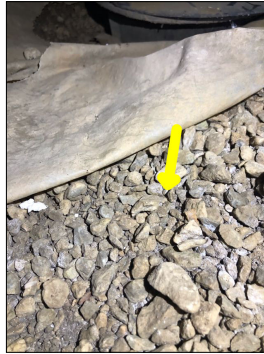
The crawl space has an exposed gravel floor in some areas that exposes the earth. Exposed gravel floors are not recommended. A gravel floor can allow the intrusion of moisture, insects, wood destroying insects, radon, mice, and rodents. An active or intermittent water source can cause mold growth and property damage, such as wood rot damage. It is recommended that the crawl space be properly encapsulated.
