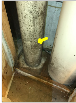
Mold like substance along the water softener. An active or intermittent water source can cause mold growth and property damage.
