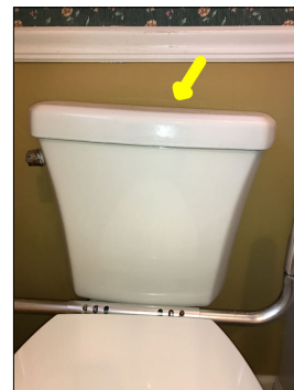
The toilet is crooked/slanted. This is considered abnormal and amateur craftsmanship. A crooked toilet is considered a cosmetic defect.
