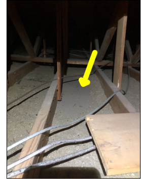
There is no insulation along the attic floor area that is located above the garage. This is not a recommended practice. The lack of insulation is not energy efficient and can cause the garage to drop below freezing temperature. Recommend adding insulation along the attic floor area that is above the garage.
