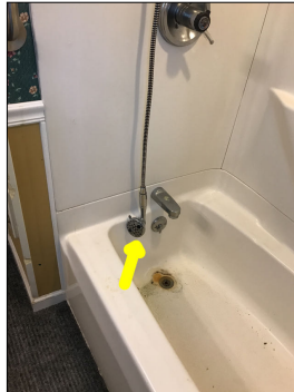
The spray hose is unconventionally just hanging from the showerhead. This is considered abnormal. The showerhead is not designed to hold up the sprayer. The sprayer should have a mounted bracket to hang on.
