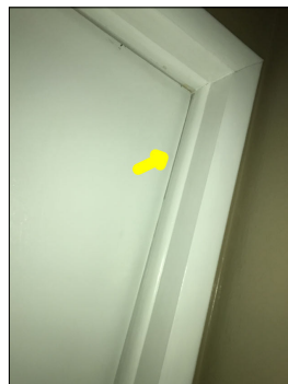
The door rubs the frame during operation.
