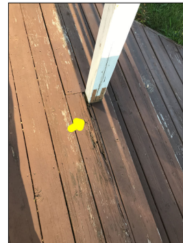
Wood rot damage.
