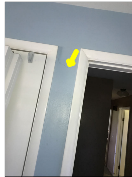
Cracks along the walls.
