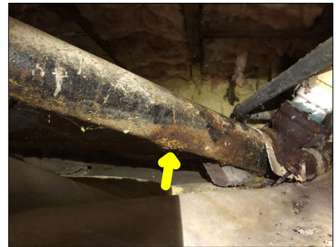
Rust, corrosion and pitting along the plumbing pipes.
