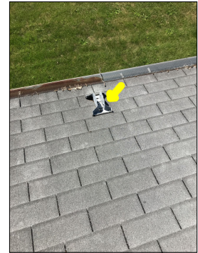
Dish brackets mounted to the roof. While mounting a dish to a roof is a common practice, it is not a recommended practice due to the anchor bolts that penetrate the roof shingles, underlayment and sheathing, thus creating a potential leak point.
