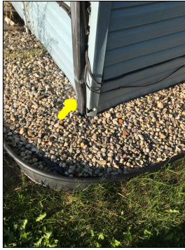
The downspout is loose.
