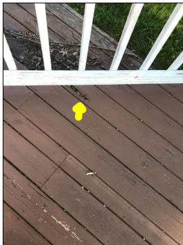
Wood rot damage.
