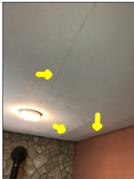
Cracks along the ceiling.
