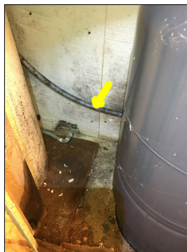
Polybutylene plumbing lines. Polybutylene pipes are prone to failure and no longer meet modern day plumbing standards. Recommend upgrading from polybutylene pipes to modern day plumbing materials, such as PEX or copper. Please note, polybutylene pipes can be concealed behind walls, ceilings, etc.
