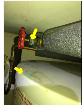
Corrosion along the water supply lines.
