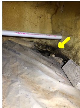
Discoloration and signs of water intrusion within the crawl space. An active or intermittent water source can cause mold growth and property damage.
