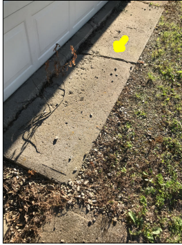
Cracks and deterioration along the driveway.
