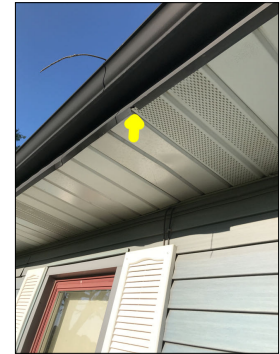
Gaps along the siding.
