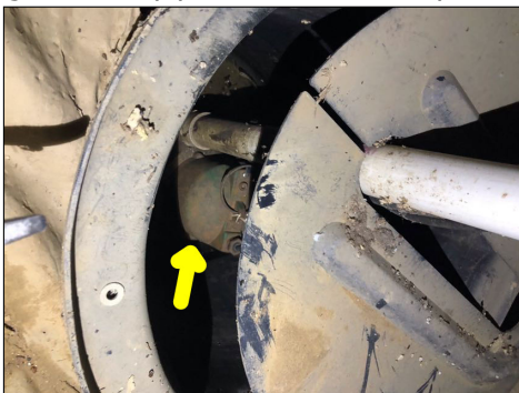
The sump pump is operable.
