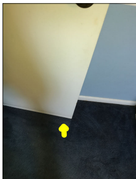
The door drags the floor during operation.
