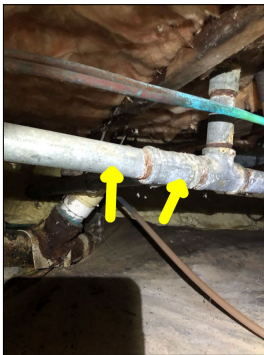
Aged galvanized water lines/pipes. Galvanized pipes no longer meet modern day plumbing standards. Galvanized pipes are prone to corroding from the inside out. Galvanized pipes are towards the end of their life expectancy. Repairs or replacement to galvanized pipes should be anticipated.
