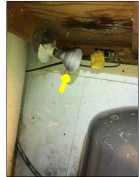
Heat lamp/bulb observed. This area might get below freezing temperatures in the winter and heat and insulation are needed to ensure water pipes and components do not freeze and burst, thus causing property damage.
