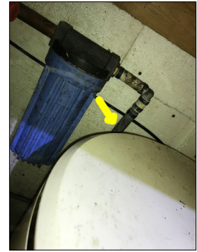
Polybutylene plumbing lines. Polybutylene pipes are prone to failure and no longer meet modern day plumbing standards. Recommend upgrading from polybutylene pipes to modern day plumbing materials, such as PEX or copper. Please note, polybutylene pipes can be concealed behind walls, ceilings, etc.
