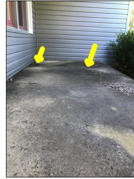
The porch slopes towards the house. This can cause water to flow towards the house, thus potentially causing water intrusion into the house and potential foundation problems due to excessive hydrostatic pressure.
