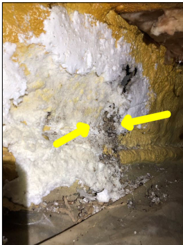
Discoloration and a foreign substance along the foundation wall. This appears to be a mold like/fungus substance. An active or intermittent water source can cause mold growth and property damage.
