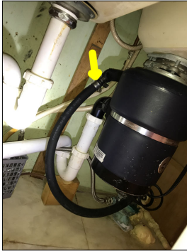
The dishwasher drain line does not have a high loop. A high loop prevents drain water from flowing into the dishwasher and contaminating the clean dishes.
