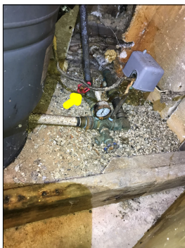
Apparent main water shut-off valve.
