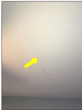
Cracks along the ceiling.
