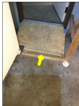
Unconventional ramp into the house. This is a potential trip hazard.
