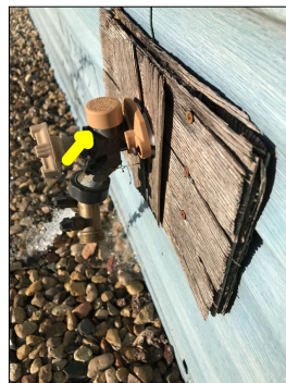
The hose bib leaks during operation. This is considered a defect.
