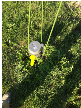
The wellhead cover is loose.
