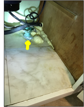
Pest control observed. Wildlife activity can cause property damage.
