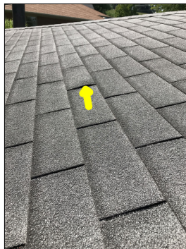
Lifted shingles. Lifted shingles are considered a defect. Lifted shingles are prone to wind damage and can allow water/moisture to get underneath them, thus creating leak points.
