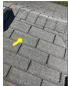
Granule loss along the roof shingles
