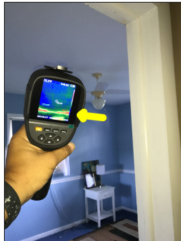
The heating elements in bedroom 1 are inoperable.
