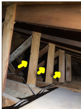
Added supports/webbing observed in the attic. This is an indication of previous structural repairs. This can be identified by the color contrast among the wood framing.
