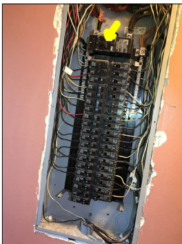
Main circuit breaker.
