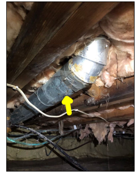
The dryer ductwork lacks insulation. This is not a recommended practice. The lack of insulation along the ductwork can allow moisture and condensation to form along the ductwork. An active or intermittent water source can cause the ductwork to rust and corrode. A water source can also cause mold growth and property damage.
