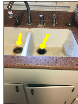
The drain is noisy. This is considered abnormal and a defect.
