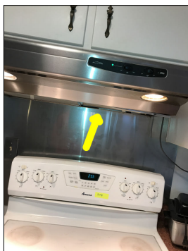
Inoperable exhaust fan.
