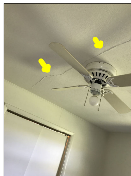
Cracks along the ceiling.
