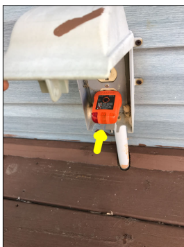
The receptacle is inoperable.
