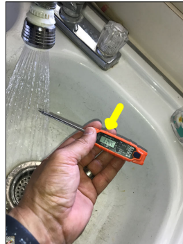
Temperature reading of the hot water during the time of the inspection. The approximate temperature of the hot water was 114 degrees Fahrenheit.
