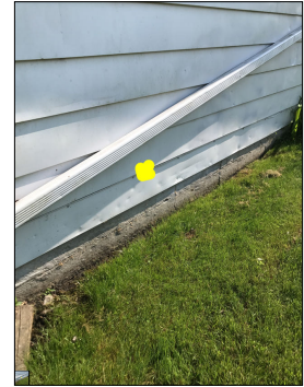
Dents along the siding.
