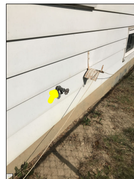
Inoperable hose bib. The hose bib is also loose.
