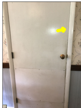
The door rubs the frame during operation.
