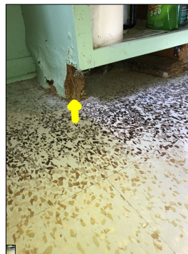
Water damage underneath the sink. An active or intermittent water source can cause mold growth and property damage, such as wood rot damage.
