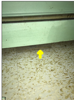
Unfinished floor/missing floor coverings.
