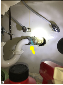
Rust/corrosion along the plumbing pipes.
