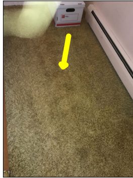
The floor slopes. This is considered abnormal and a defect.
