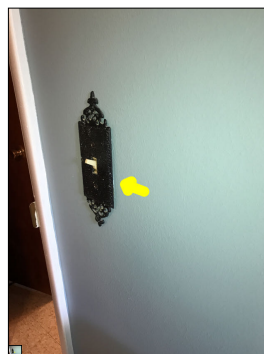
The light switch is not flush with the wall and is loose. This is considered a defect and a potential safety hazard.
