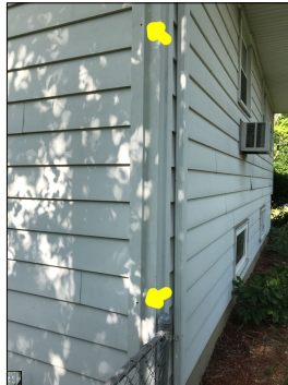
Holes along the siding.
