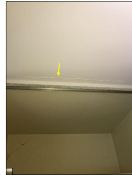
Cracks along the ceiling.
