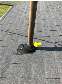
Unconventional application of roof sealant along the rubber flashing. Rubber flashing is designed to be caulkless. This is considered amateur craftsmanship. Most roof sealants are petroleum based. A petroleum based product can cause the rubber flashing to prematurely deteriorate, thus creating a leak point.
