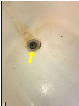
The drain is missing a grate/screen. The lack of a grate/screen over the drain can allow debris down the drain, thus potentially creating slow drainage or blockage.
