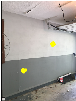
Cracks along the walls.
