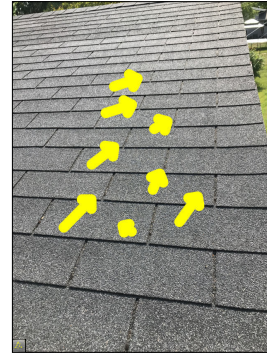
The 3 tab roof shingle cutouts align every other course. Some shingle manufacturer specifications for installation prohibit cutouts to align every other course. The alignment of cutouts every other course can cause premature weathering of surface granules. When cutouts are staggered, runoff is less likely to cut channels into the shingle granules. Also, staggered cutouts better hide shingle irregularities and discoloration from different shingle lot numbers.
