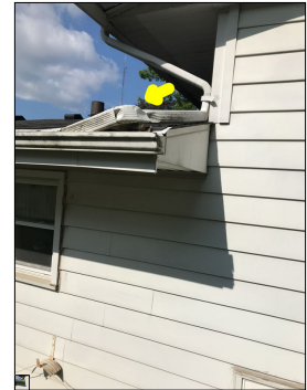
Dents/damage along the gutter system.
