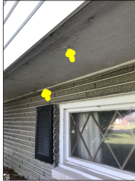
Flaking and peeling along the siding.
