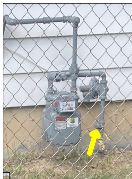
Main fuel shut off valve.
