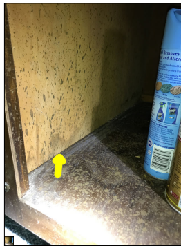
Signs of previous water damage underneath the sink and a mold like substance. An active or intermittent water source can cause mold growth and property damage, such as wood rot damage.
