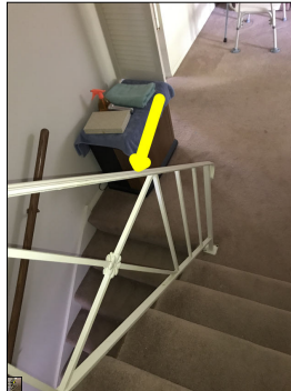
The handrail is loose.
