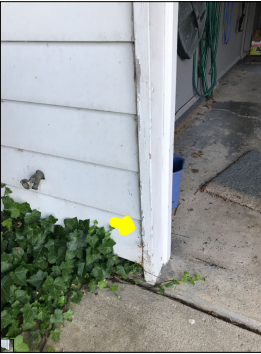
Flaking and peeling along the siding.
