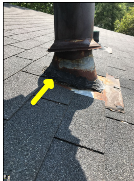
Unconventional application of sealant along the roof. This is considered abnormal and amateur craftsmanship. Amateur craftsmanship is prone to failure and leakage.
