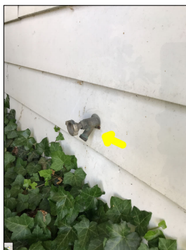
No anti-siphon/frost free valve. The lack of an anti-siphon valve can allow water back flow into the water supply lines, thus contaminating potable water. This is a potential safety hazard. The lack of a frost free valve can allow water to stay within the hose bib, which could potentially freeze during cold months and cause the pipe to rupture. This can cause property damage.
