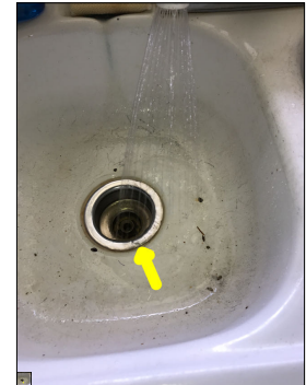
The drain is noisy. This is considered abnormal and a defect.
