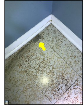
Deterioration along the floor covering.
