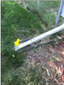
Dents/damage along the gutter system. The downspout is smashed.
