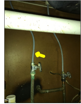
Polybutylene plumbing lines. Polybutylene pipes are prone to failure and no longer meet modern day plumbing standards. Recommend upgrading from polybutylene pipes to modern day plumbing materials, such as PEX or copper. Please note, polybutylene pipes can be concealed behind walls, ceilings, etc.
