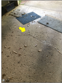
Cracks and deterioration along the floor.
