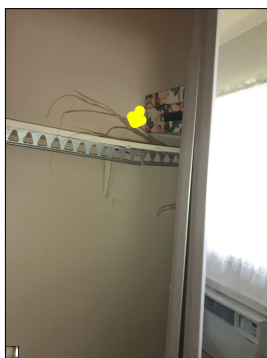
Broken shelf in the closet.
