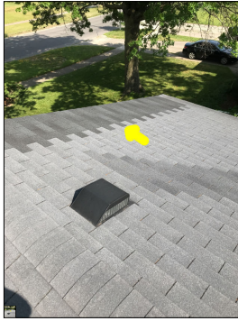
Previous repairs along the roof shingles. Also, the shingle colors do not match.
