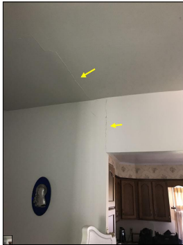
Cracks along the walls and ceiling.
