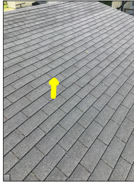
The roof decking is spongy. There are areas along the roof that sag and move while walking the roof. This is considered abnormal and a defect.
