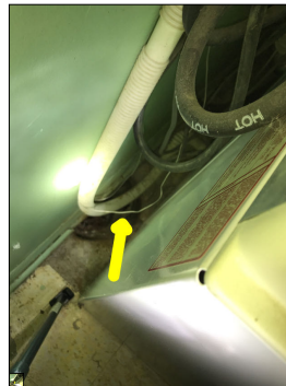
Unconventional hole/floor drain located behind the washer. The location of the hole/drain is odd. The hole can allow radon gas, moisture, and potentially abnormal smells into the house.
