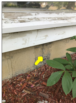
Crack along the foundation. Cracks are considered a defect. Cracks should be repaired/sealed to prevent the intrusion of moisture, insects, wood destroying insects, mice, and radon.
