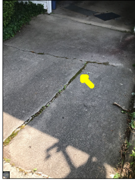
Cracks and deterioration along the driveway.
