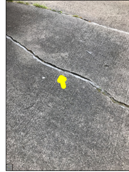
Uneven surfaces along the driveway.
