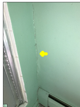
Flaking and peeling along the walls.
