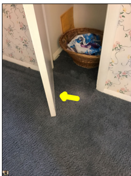
The door drags the floor during operation.
