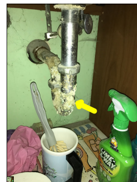
Rust/corrosion along the plumbing pipes.
