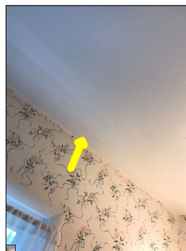
Discoloration along the ceiling.
