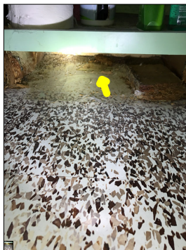
Active plumbing leak. An active or intermittent water source can cause mold growth and property damage.
