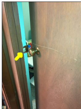
The door does not latch properly.
