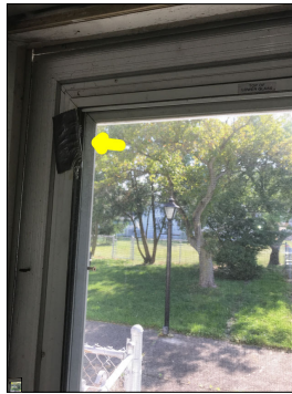
The glass insert is loose.
