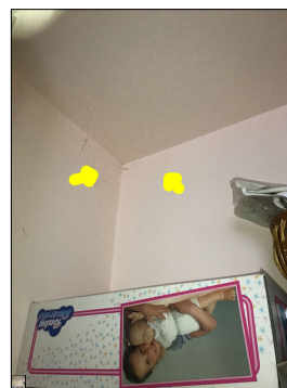
Flaking and peeling along the walls.
