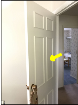
The door rubs the frame during operation. The door does not stay open.
