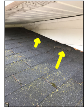
Loose/detached roof shingles. This is considered a defect and a potential leak point.
