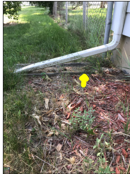
The splash block is sloped towards the house. This can cause water to flow towards the house.
