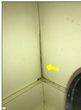
Cracks and damage along the walls.
