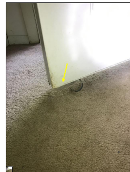
Torn weatherstrip along the door.
