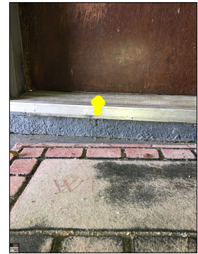
Daylight can be seen from the interior. This is an entry point for moisture, insects, mice, rodents, etc.
