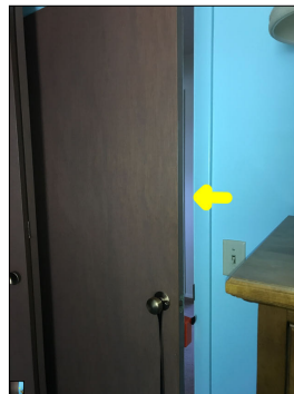
The door does not latch properly.
