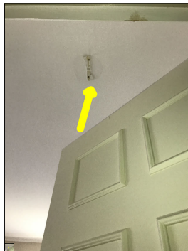
Missing smoke detector. There are several missing throughout the house.
