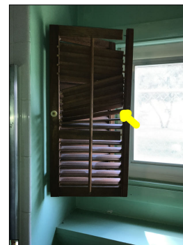
Damaged window coverings.
