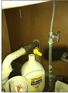
Aged copper drain pipes. Copper pipes make good water supply lines, however, they are not as effective for drain pipes. This is because copper drain pipes are thin walled, which means they are not very robust. Also, some cleaning products and house hold products are acidic which causes copper pipes to corrode. Also, urine is acidic, which can also cause copper pipes to corrode. Due to the age of copper drain pipes, repairs should be anticipated and possible replacement of copper drain pipes should be anticipated.
