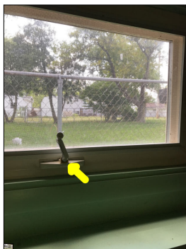
The window is difficult to operate.
