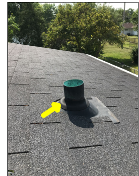
The plumbing vent is unconventionally short. This is considered abnormal and a defect. A short plumbing vent can get covered during heavy snowfall, thus obstructing the vent, which could result in drainage problems with the plumbing system.
