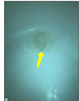
The bathtub has been resealed. This is an indication that the bathtub required maintenance and/or repairs. Long-lasting repair to a bathtub is difficult to achieve. Bathtubs are designed to hold water and making water tight and leak proof repairs is difficult to achieve. Additional repairs to a recently repaired bathtub should be anticipated in the near future.
