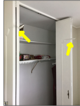
Unconventional trim sticking out from the doors.
