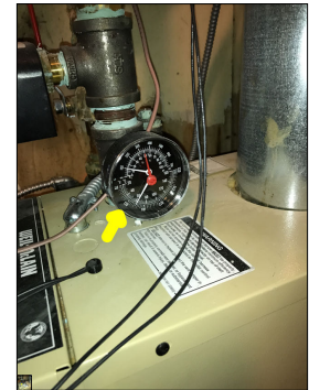
General photo of the temperature and pressure gauge.
