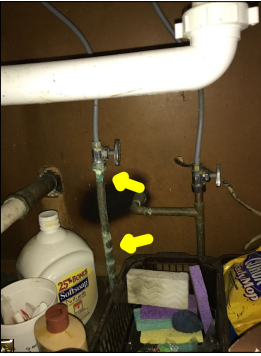
Rust/corrosion along the plumbing pipes.
