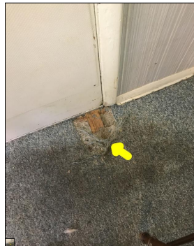
Damaged floor coverings.
