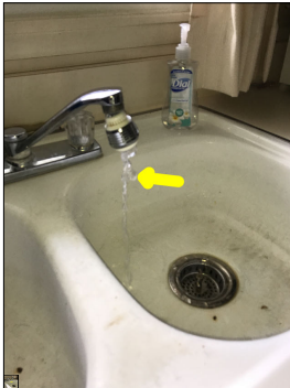
Abnormal water pressure/flow from the faucet. The spray pattern alternates. The wide spray pattern sprays water outside the sink basin.
