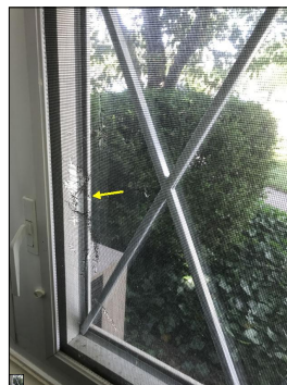
Holes along the window screen.
