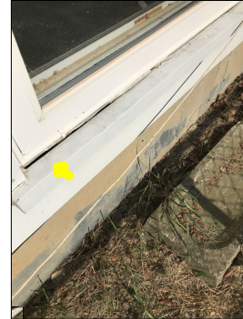
Gaps along the siding.
