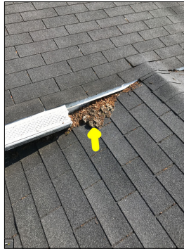
Debris along the roof. Excessive debris along the roof can restrict the ability of the roof to shed water, thus creating potential leak points.
