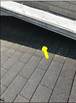
Biological growth along the roof. This is considered a defect. Biological growth has the potential to hold water. Shingles are not designed to hold water, shingles are designed to shed water.
