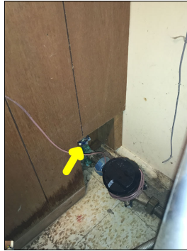
Main water shut off valve.
