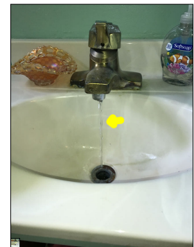
Abnormal water pressure/flow from the faucet.
