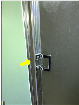
The door does not latch.
