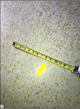
9" X 9" floor tiles. These tiles are potential asbestos based tiles. Asbestos based products are considered a potential health/safety hazard.
