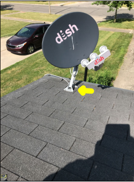
Dish mounted to the roof. While mounting a dish to a roof is a common practice, it is not a recommended practice due to the anchor bolts that penetrate the roof shingles, underlayment and sheathing, thus creating a potential leak point.
