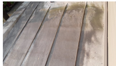
Water staining which indicates water pooling in the area
