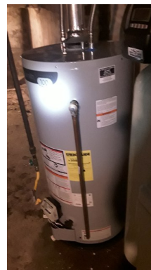
water heaters should not be placed on the ground. The should be on a barrier from moisture in cement.
