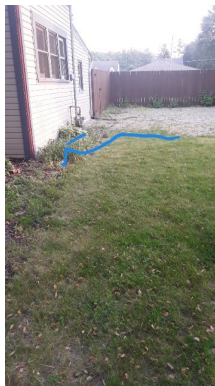
some erosion in this area.
