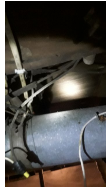
I found this in the basement. It's a normal house wire feeding into a knob and tube the white wire which is actually connected to the knob and tube is not hot. Which makes the knob and tube not hot. The hot wire does have a cap on it however any splice should be in a junction or protective box
