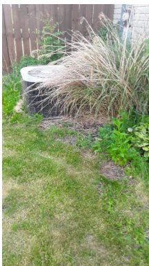
green growth can get into the fan of the AC unit.
