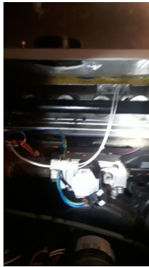
Wires outside of a junction box
