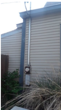
heavy rust on the meter cover.
