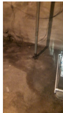
Heavy rest to the bottom for Jack support. The floor is currently wet during time of inspection
