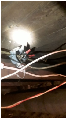
any wire splice connection should be in a junctional box.
