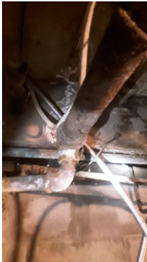
heavy rust to the gas line.
