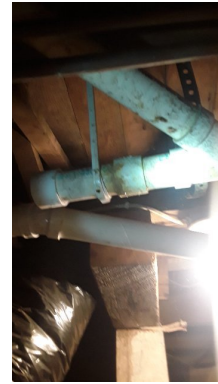
it is wet at the connection. water will sit in this spot due to the way it is designed. Really not a huge concern unless it continues to seep.
