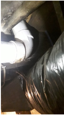
This is coming from downstairs toilet
