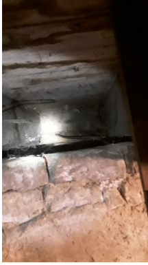
area with heavy discoloration to the subflooring
