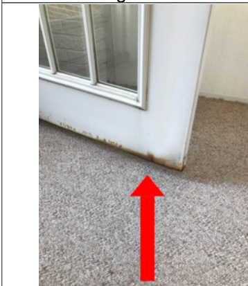
Water damage along the entry door.
