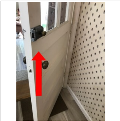
The door latch is inoperable.
