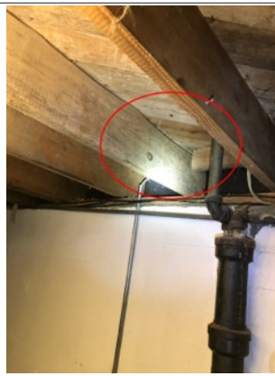
The top of the floor joist is partially missing. This is considered abnormal. Also, there is discoloration along some areas of the subfloor and floor joists. Discoloration can potentially be a mold like substance.
