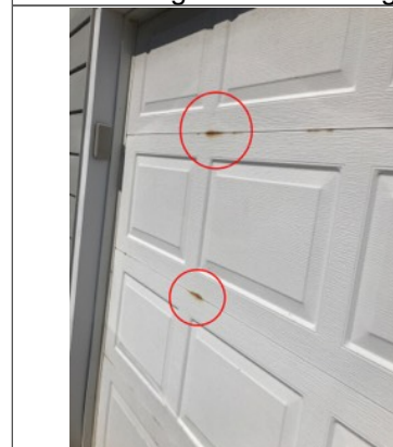
Rust/corrosion along the overhead garage door.
