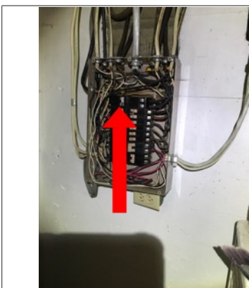
Main circuit breaker.
