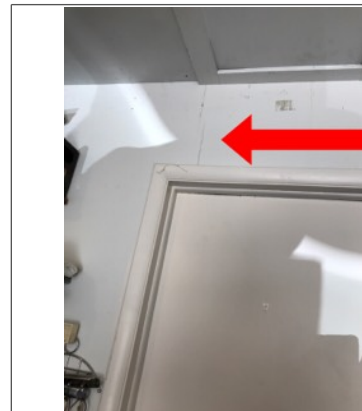
Cracks along the walls/ceiling.
