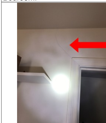
Cracks along the walls/ceiling.
