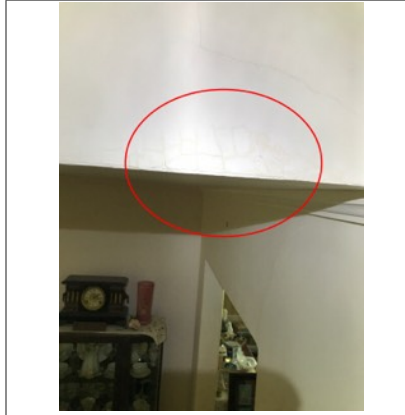
Cracking/flaking along the wall.
