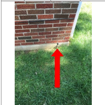
Cracks along the foundation.
