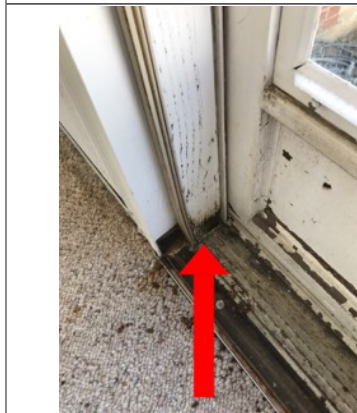
Wood rot damage along the door frame.
