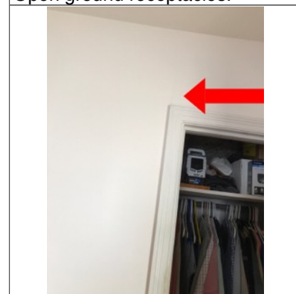
Crack along the wall.
