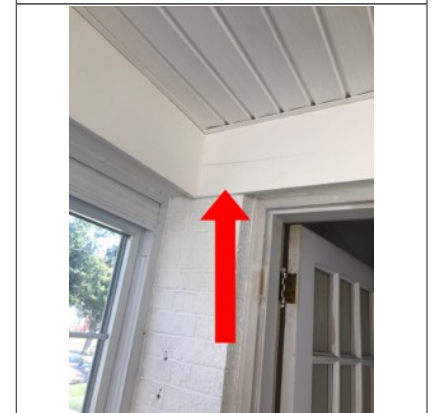
Crack along the wall.
