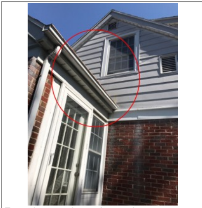
Rust/corrosion along the gutter system and dents.
