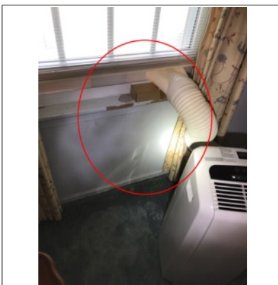
Cracks along the wall and flaking/peeling along the window sill.
