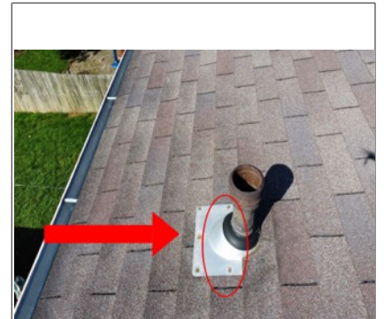
The flashing is not properly tucked underneath the shingles. This is considered amateur craftsmanship. Amateur craftsmanship is prone to failure and leakage. The flashing should also be tucked underneath the middle layer of shingles that is identified by the circle in the photo.
