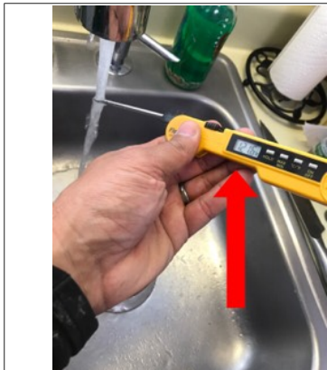
Temperature reading of the hot water during the time of the inspection. The approximate temperature of the hot water was 121 degrees Fahrenheit.
