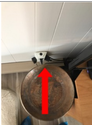
There is a receptacle above the electric baseboard. This is a potential safety hazard. An electrical cord could come in contact with the baseboard. This can cause overheating, spark and potential fire.
