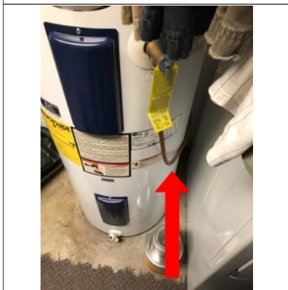
Defects with the temperature and pressure relief valve extension. The temperature and pressure relief valve extension should not have any bends and should be within 6 inches from the floor.
