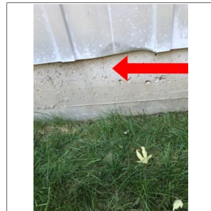
Crack along the slab.
