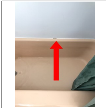
Missing caulk. This is a leak point for water to get behind the wall.
