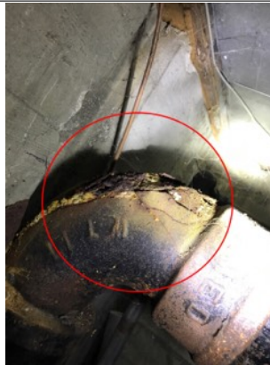
Aged/corroded cast iron drain pipes.
