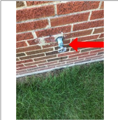
No anti-siphon/frost free valve.
