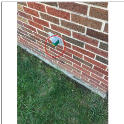
Non GFCI protected receptacles.
