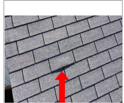
Lifted roof shingles. Lifted shingles are prone to wind damage and are leak points as water can get underneath them.
