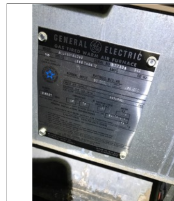
Furnace data plate.
