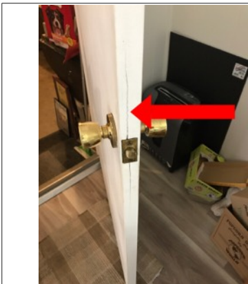
The door is split.
