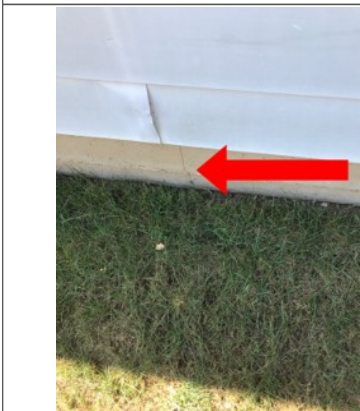
Crack along the slab.
