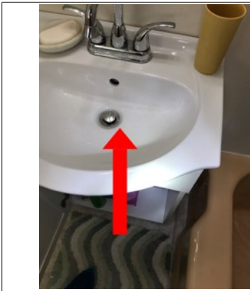
The drain makes a gurgling sound.
