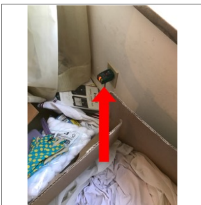
Open ground receptacles.
