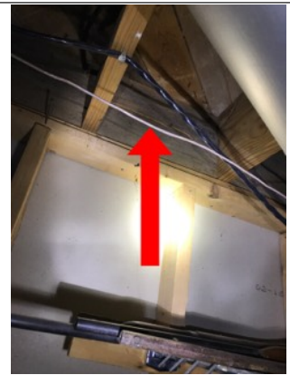
Cracked band joist.
