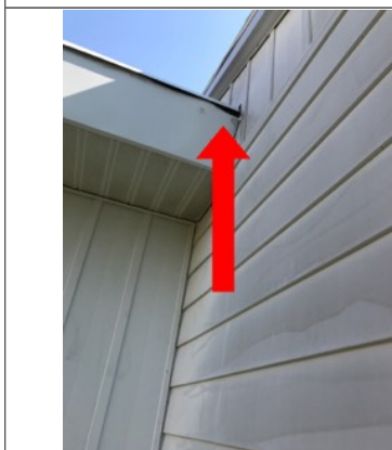
Gap along the siding.
