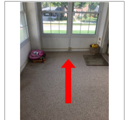
The floor slopes.
