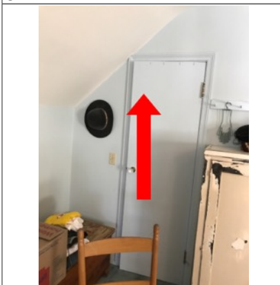
The door does not latch properly.
