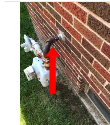
Rust/corrosion along the fuel lines. Excessive rust/corrosion can cause holes in the lines, thus creating a fuel leak.
