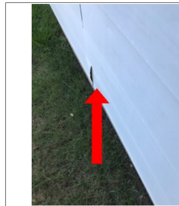
Gap along the siding.
