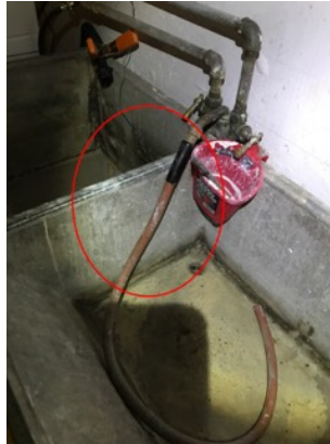
The drain is noisy.
