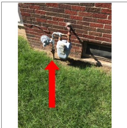
Main fuel shut off valve.
