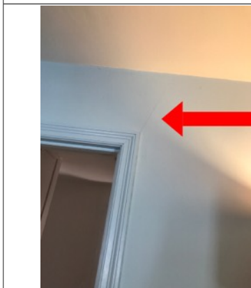
Crack along the wall.
