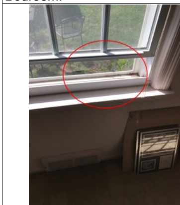
Torn window screen.
