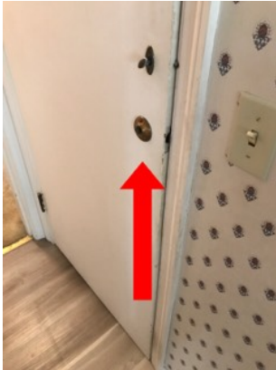
Handle is missing to the door to the basement.
