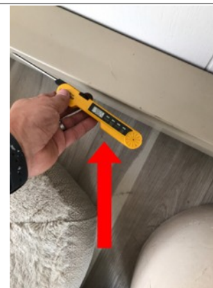
The electric baseboards are operable.
