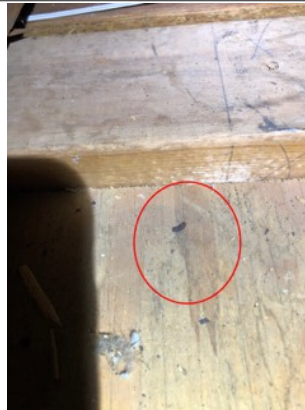
Mice/rodent droppings within the attic.
