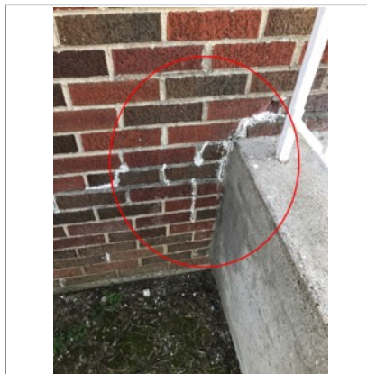
Cracks along the brick siding with signs of amateur repairs. Someone applied some caulk along the brick and mortar.
