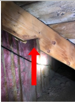
Unconventional notch along the truss.
