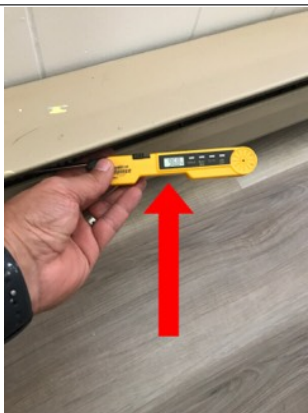
The electric baseboards are operable.
