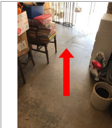
Cracks along the floor.
