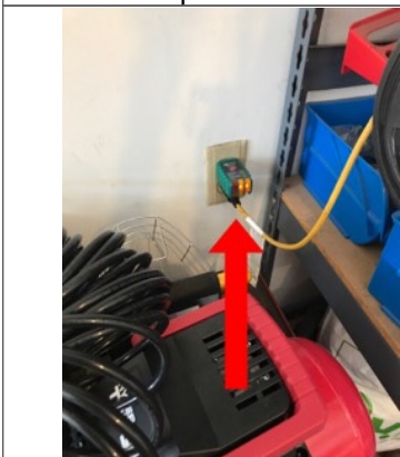
Non GFCI protected receptacles.
