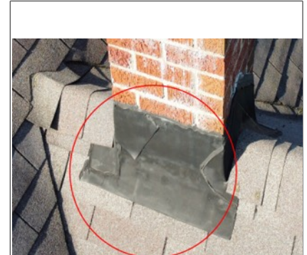
Unconventional flashing around the base of the chimney. The flashing is considered amateur craftsmanship. Amateur craftsmanship is prone to failure and leakage.
