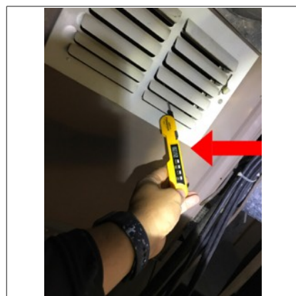
The photo identifies the temperature of the supply air while the air conditioner was in operation. The approximate temperature of the supply air was 48 degrees Fahrenheit.
