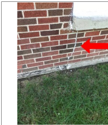
Crack along the brick siding.
