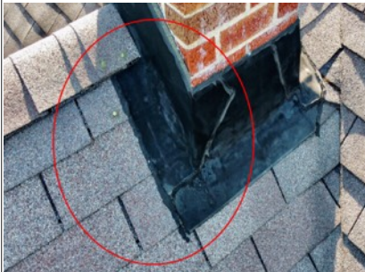
Exposed nailheads and unconventional flashing. Exposed nailheads are potential leak points. The flashing is unconventionally sitting on top of the shingles. This is considered amateur craftsmanship. Amateur craftsmanship is prone to failure and leakage.
