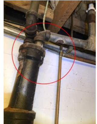
Aged corroded cast iron drain pipes.
