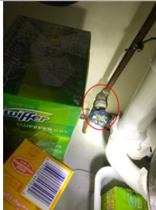
Corrosion along the water supply lines. This is located underneath the sink.
