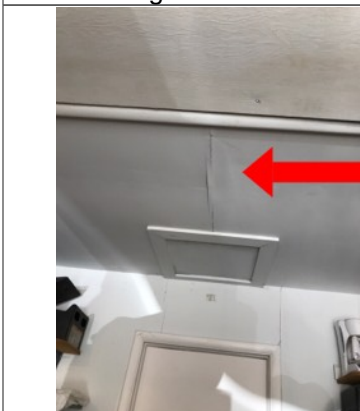
Cracks along the ceiling.
