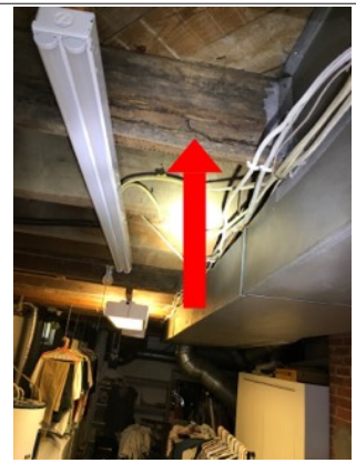
Cracked floor joist.
