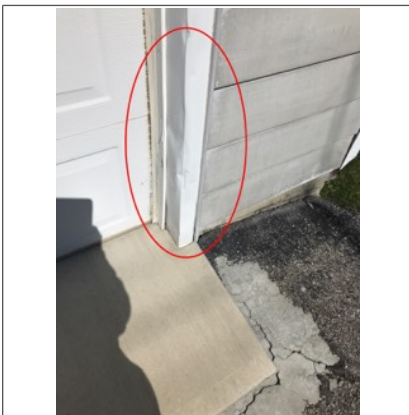
Dents along the capping.
