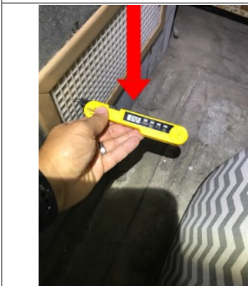
The photo identifies the temperature of the return air while the air conditioner was in operation. The approximate temperature of the return air was 64 degrees Fahrenheit.
