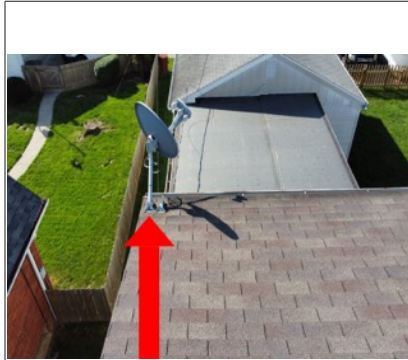
Dish mounted to the roof. While mounting a dish to a roof is a common practice, it is not a recommended practice due to the anchor bolts that penetrate the roof shingles, underlayment and sheathing thus creating a potential leak point.
