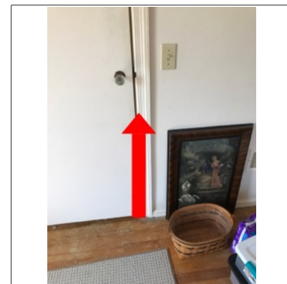
The door does not latch properly.
