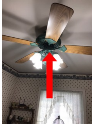
The ceiling fan is inoperable.
