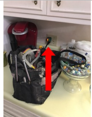
Open ground receptacles. Also, the receptacles are non GFCI protected.
