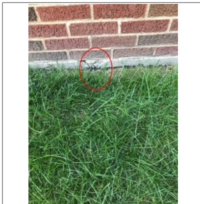
Deterioration along the foundation.
