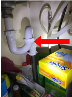
S-trap underneath the sink. S-traps no longer meet modern day plumbing standards. S-traps have the potential to siphon and become dry thus creating the potential to allow sewer gases into the house. S-traps also have the potential to make a knocking/gurgling sound when draining.
