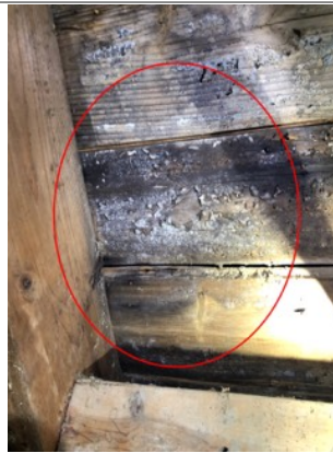
Mold like substance along the sheathing. An active or intermittent water source can cause mold growth, discoloration, and wood rot. The mold like substance covers the majority of the attic sheathing.
