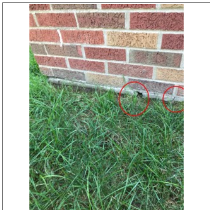
Crack/deterioration/gap along the foundation. Areas such as these should be monitored for signs of additional movement. This area should be filled with an exterior grade adhesive or concrete to prevent the intrusion of mice, insects, rodents, moisture, etc.
