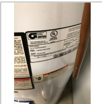
Water heater data plate.
