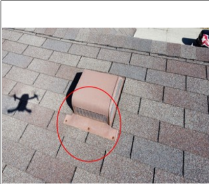
Exposed nailheads. Exposed nailheads are potential leak points.
