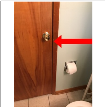
The door does not latch properly.
