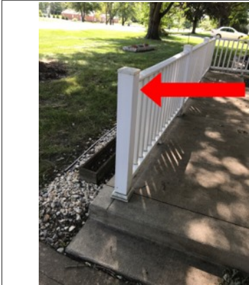
The railing is loose.
