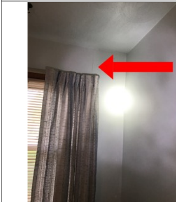
Cracks along the walls.
