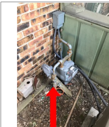
Main fuel shut off valve.
