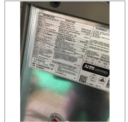
Furnace data plate.
