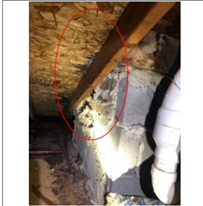
Signs of previous water intrusion along the sheathing and mold like substance. An active or intermittent water source can cause mold growth and wood rot. This is adjacent to the chimney.
