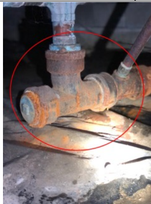
Aged/corroded cast iron drain pipes within the crawl space. Water was observed underneath the pipe. The cast iron drain pipes are at the end of their lifespan and should be replaced.
