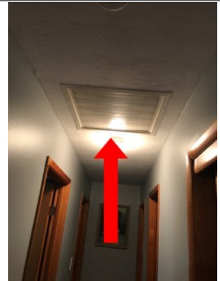
The whole house attic fan is operable.
