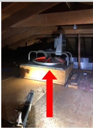
There is a whole house fan in the attic.
