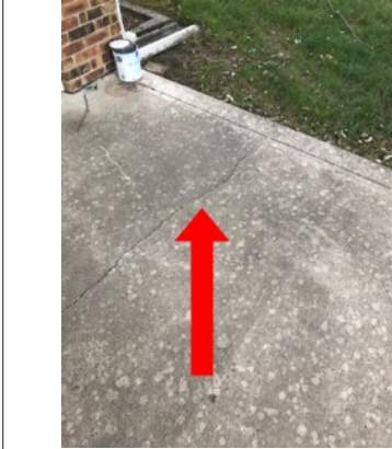
Cracks along the driveway.
