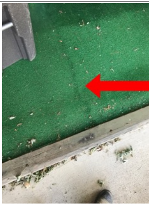
Uneven surfaces along the floor.
