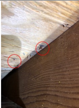
Some nails along the sheathing are rusty. This is an indication that the nails have been exposed to moisture and/high levels of humidity. Inadequate ventilation and insulation can cause condensation to form on the nails. An active or intermittent water source can cause mold growth and structural damage, such as wood rot.
