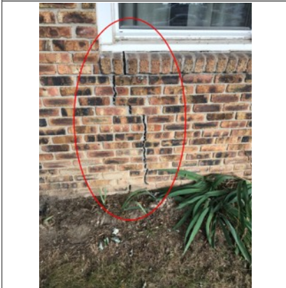
Cracks along the siding.
