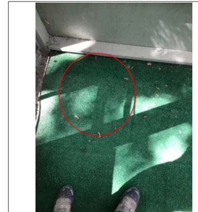
Uneven surfaces along the floor.
