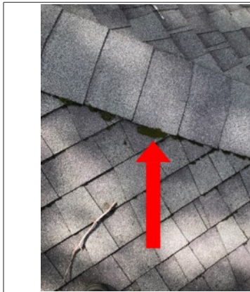
Biological growth along the roof. Biological growth has the potential to hold water, thus creating potential leak points.
