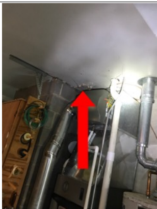
Damage along the ceiling.
