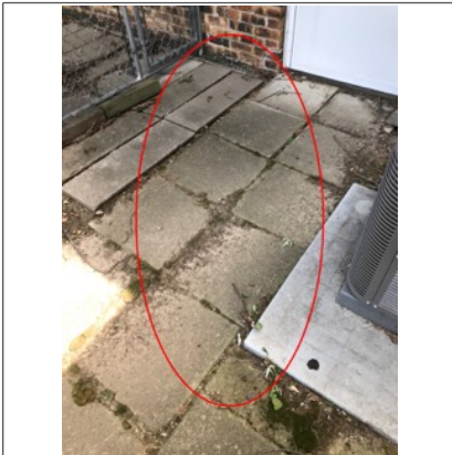
Uneven surfaces along the service walks.
