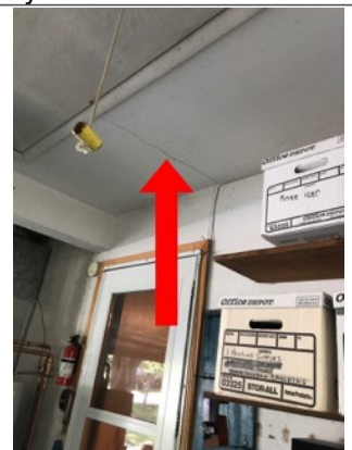
Cracks along the ceiling.
