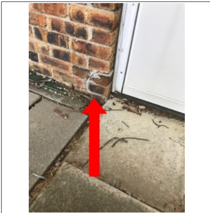
Cracks along the siding.
