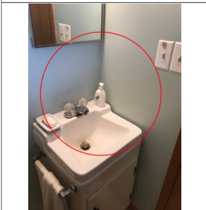
There are no apparent receptacles in the bathroom.
