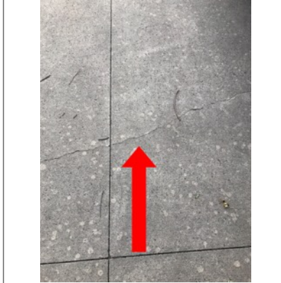
Cracks along the driveway.
