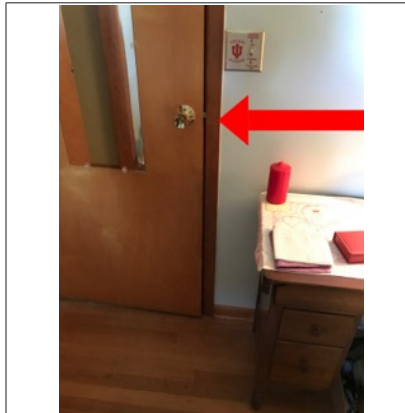
The door does not latch properly.
