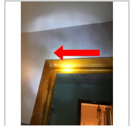
Cracks along the wall.
