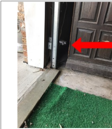
The photo eye sensors are too high. They should be between 4 to 6 inches from the floor.
