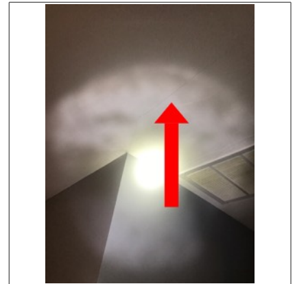
Cracks along the ceiling.
