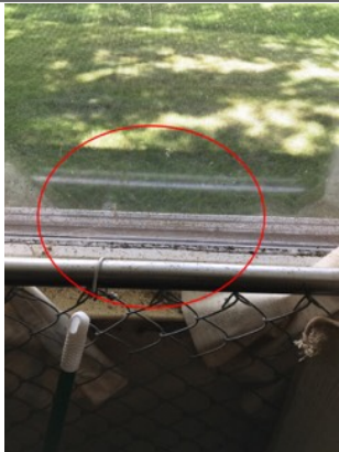
Mold like substance along the window. An active or intermittent water source can cause mold growth.
