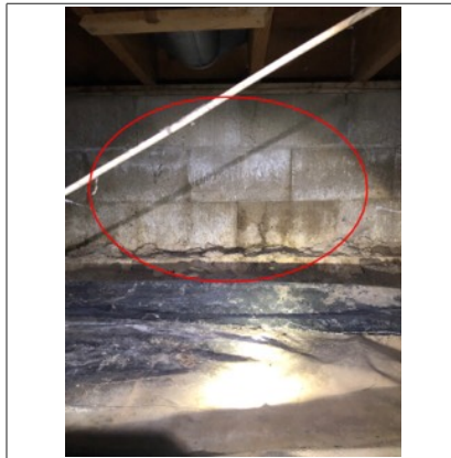
Efflorescence and signs of previous water intrusion.
