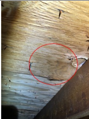
Some areas along the sheathing are delaminated.
