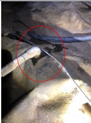
The condensation line from the air conditioning/furnace is discharging on the floor. This is considered amateur craftsmanship. An active or intermittent water source can cause mold growth.
