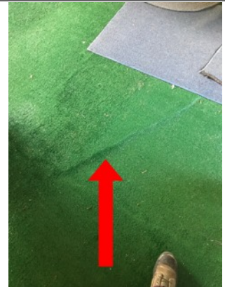
Uneven surfaces along the floor.
