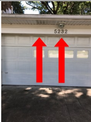
The header unconventionally sags in the middle.
