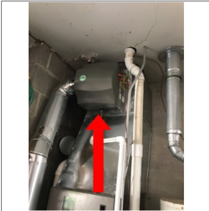
The whole house humidifier is operable.
