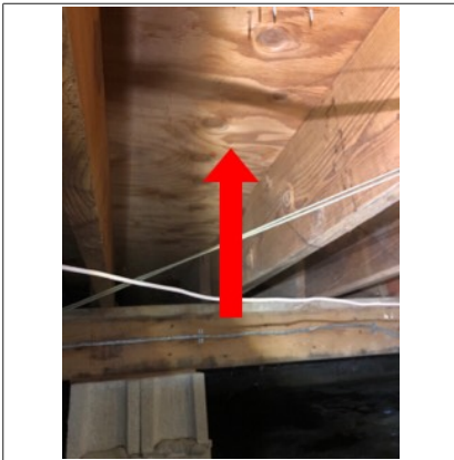
There is no insulation within the crawl space.
