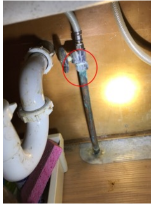
Corrosion along the water supply lines. This is located underneath the sink.
