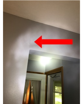
Cracks along the wall.
