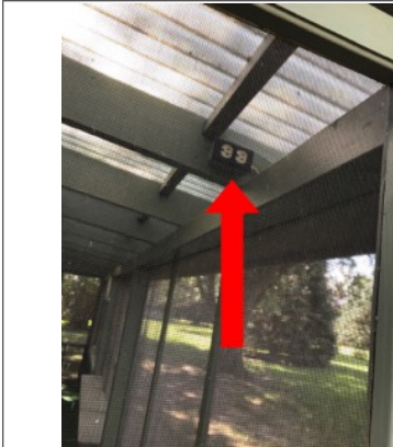
The exterior receptacle is missing a weather protection cover.
