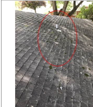
Biological growth along the roof. Biological growth has the potential to hold water, thus creating potential leak points.
