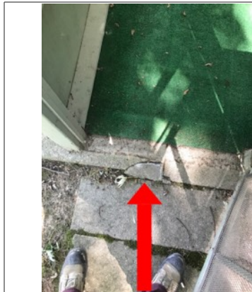
Cracks and deterioration along the floor.
