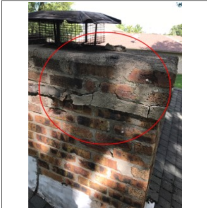
Deterioration along the brick and mortar.
