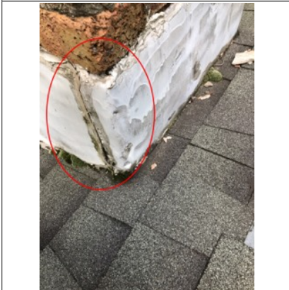
Gaps along the flashing. Gaps are potential leak points.
