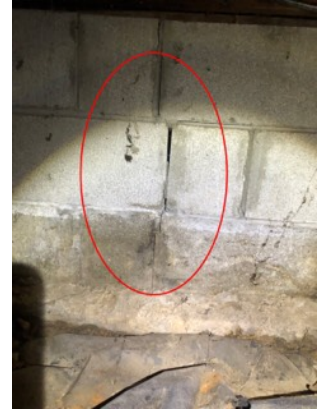
Cracks and deterioration along the foundation walls.
