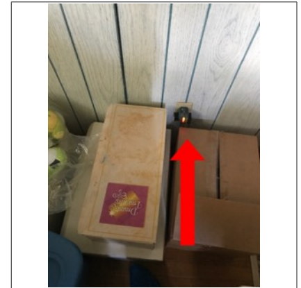
Open ground receptacles.
