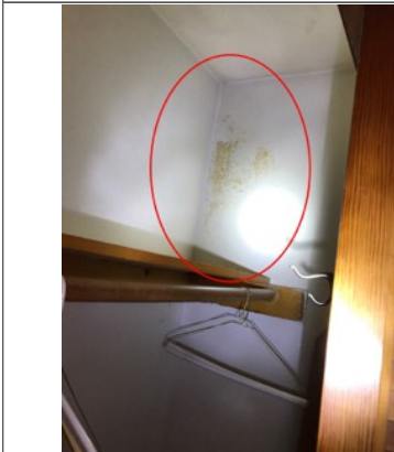
Discoloration/mold like substance along the wall. An active or intermittent water source can cause mold growth.
