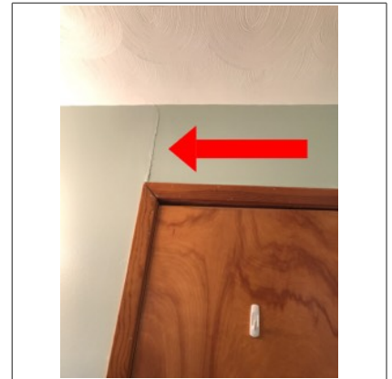
Cracks along the walls.
