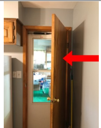
Improper door that separates the interior of the house from the garage. The door is a hollow door and is not properly fire rated. The hollow door is a potential safety hazard.
