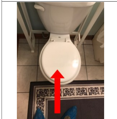
The toilet is loose. The toilet rocks from side to side. A properly installed toilet should be fully anchored to the floor and have no movement.
