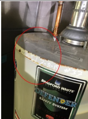
Rust/corrosion along the water heater.
