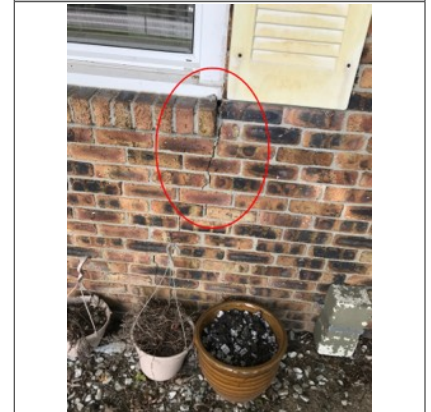
Cracks along the siding.
