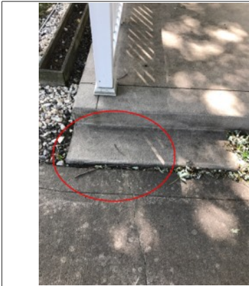
Uneven surfaces along the porch. This is a potential safety hazard.
