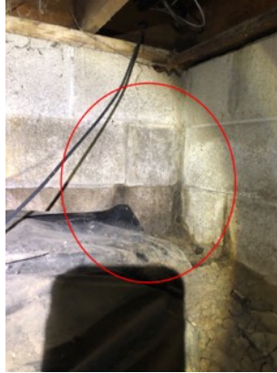
Efflorescence and signs of water intrusion within the crawl space.
