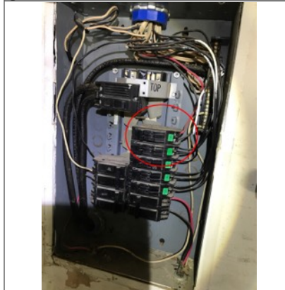
According to the wire diagram on the panel, there are tandem "twin" circuit breakers located in improper areas along the busbar. This is a potential safety hazard.
