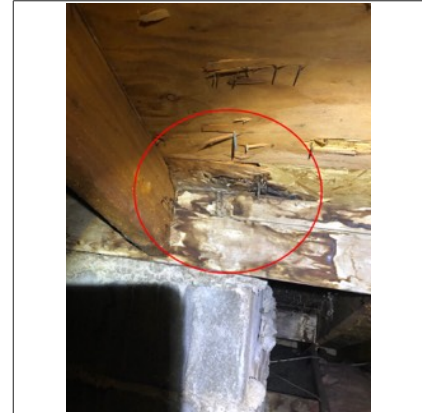
Signs of previous water intrusion along the sheathing and mold like substance. An active or intermittent water source can cause mold growth and wood rot. This is adjacent to the chimney.
