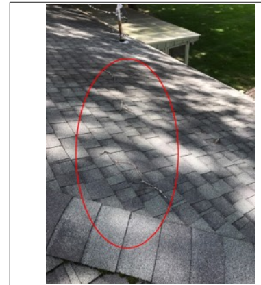
Debris and branches along the roof shingles. Falling tree branches can damage the roof shingles.
