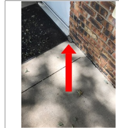
Cracks/deterioration along the porch.
