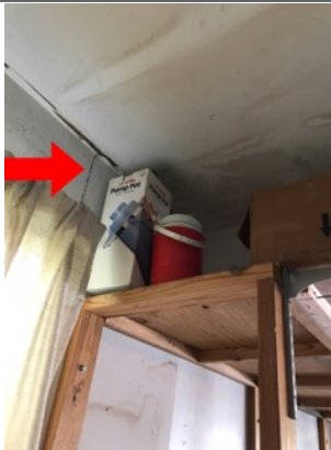
Cracks along the walls.
