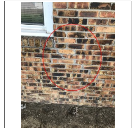
Cracks along the siding.
