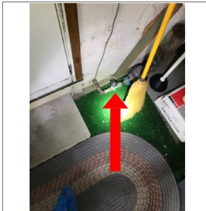
Main water shut off valve.
