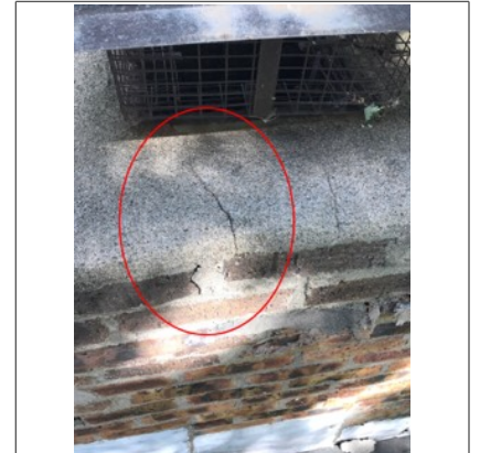
Cracks along the chimney top plate. Cracks are potential leak points.
