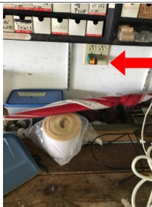
The receptacles are non GFCI protected.
