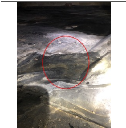
Areas of standing water within the crawl space. An active or intermittent water source can cause mold growth.
