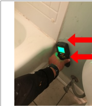
Damage along the wall and moisture detected. An active or intermittent water source can cause mold growth and structural damage, such as wood rot.
