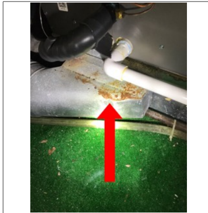
Rust/corrosion along the ductwork.
