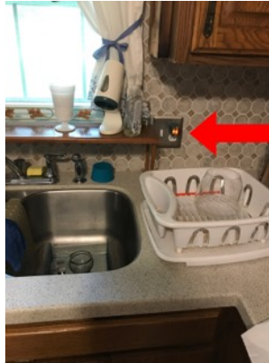
The receptacles are non GFCI protected.
