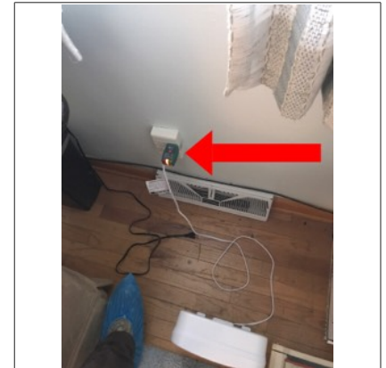
Open ground receptacles.
