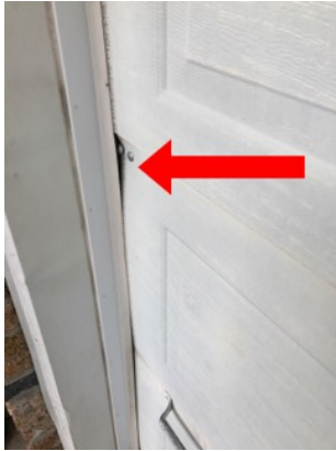
Dents along the overhead garage door.
