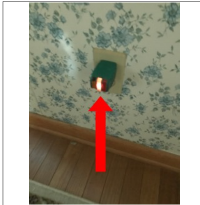
Open ground receptacles.
