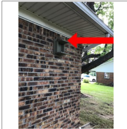
Birds nest. Birds can cause property damage if they are not properly controlled.
