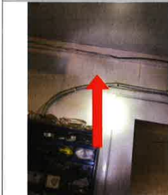
Cracks along the wall.
