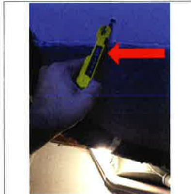
The photo identifies the temperature of the supply air while the furnace was in operation. The approximate temperature of the supply air was 102 degrees Fahrenheit.
