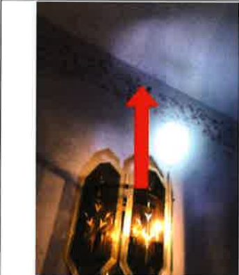
Slight cracking along the ceiling.
