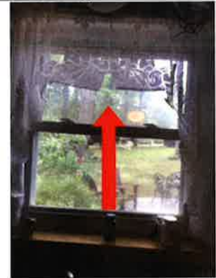
The top sash falls upon opening the window. This is considered a defect.
