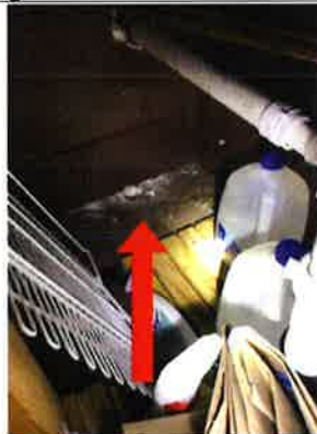
Cracks along the slab.
