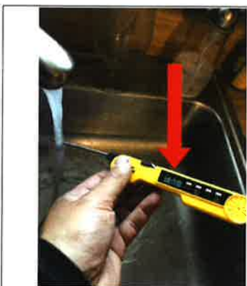
Temperature reading of the hot water during the time of the inspection. The approximate temperature of the hot water was 116 degrees Fahrenheit.
