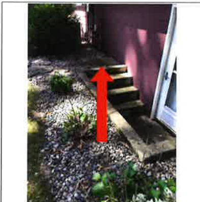
The steps do not have a handrail.
