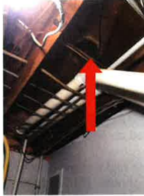
Aged copper drain/waste pipes. Copper pipes make good water supply lines, however, they are not as effective for drain/waste pipes due to some cleaning chemicals and house hold products are acidic which causes them to corrode. Also, urine is acidic which can also cause copper pipes to corrode.
