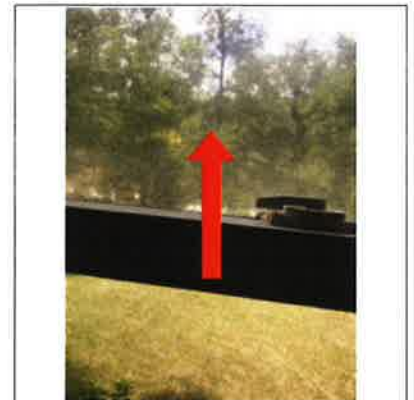
Insulated glass seal failure.
