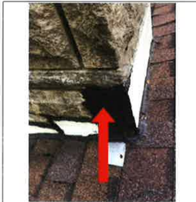
Excessive and unconventional application of sealant/caulk. This is considered amateur craftsmanship.
