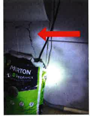
Crack along the foundation wall.
