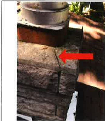
Crack along the chimney top. Cracks are potential leak points.
