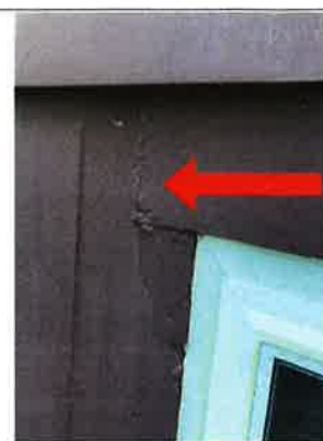
Crack along the foundation wall.
