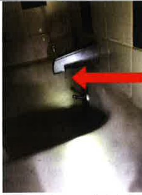
The bathtub faucet slightly leaks while the showerhead is in operation. A properly functioning diverter will not allow any water through the bathtub faucet while the showerhead is in operation.
