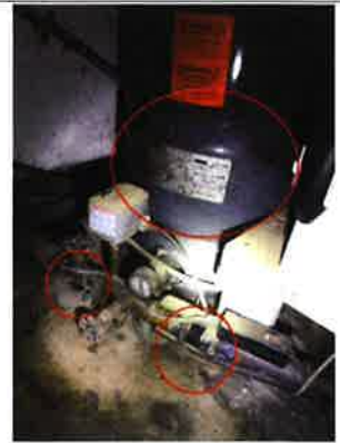
Moisture observed along the water lines and pressure tank. This is most likely condensation. It can be difficult to distinguish condensation from a leak. Due to the location of the pressure tank being in the garage, it will most likely always form condensation along it. Especially, during the warmer months. The black substance along the tank is probable mold like substance.
