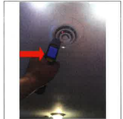
The photo identifies the temperature of the supply air while the air conditioner was in operation. The approximate temperature of the supply air was 59 degrees Fahrenheit.
