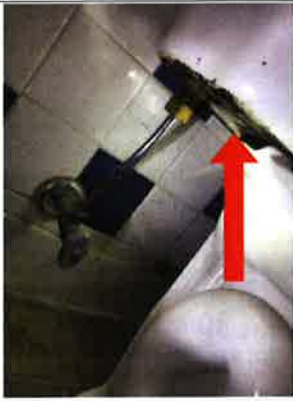
Mold like substance along the bottom of the toilet.
