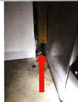
Signs of previous moisture damage underneath the dishwasher. No moisture detected during the inspection. An active or intermittent water source can cause mold growth.
