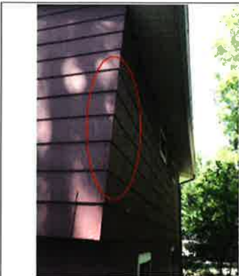
Holes along the siding.
