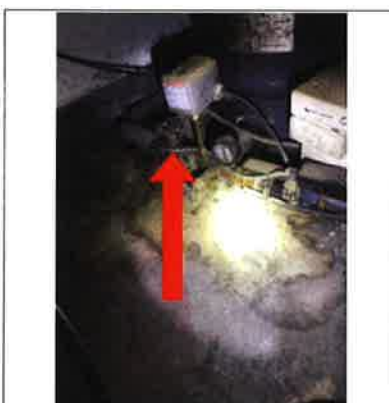
Apparent main water shut off valve.
