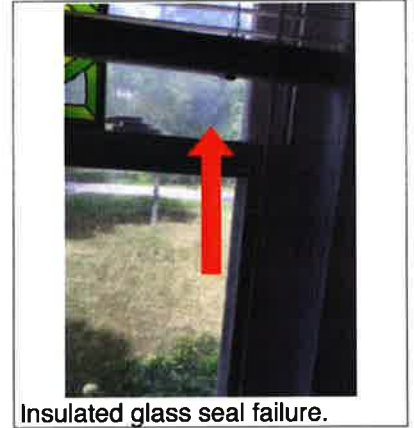
Insulated glass seal failure.
