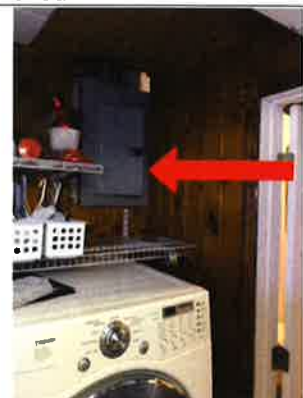
The circuit breaker panel is not readily accessible. It is recommended that circuit breaker panels be readily accessible. The recommended clearance is 36" in front and 30" side-to-side.
