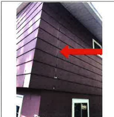
Discoloration along the siding.
