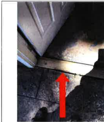
Damage along the threshold.
