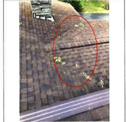
Debris along the roof.
