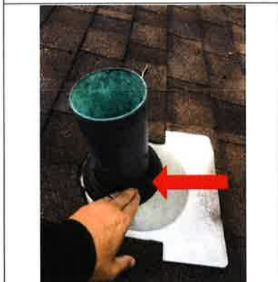
The flashing around the vent is concave. This will act as a catch for water, thus becoming a potential leak point. Flashing is not designed to hold water, flashing is designed to shed water.
