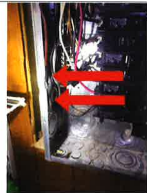
Loose unused wires. Ideally, loose/unused wires should be removed.
