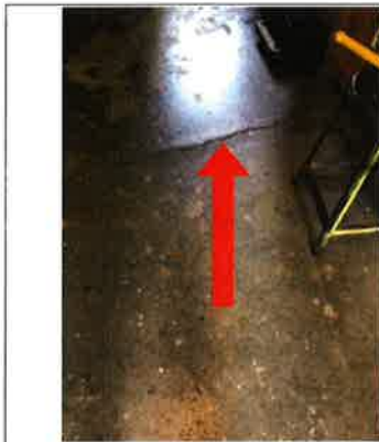
Cracks along the floor.
