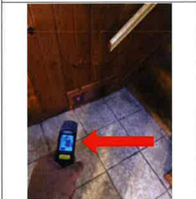
The photo identifies the temperature of the return air while the furnace was in operation. The approximate temperature of the return air was 70 degrees Fahrenheit.
