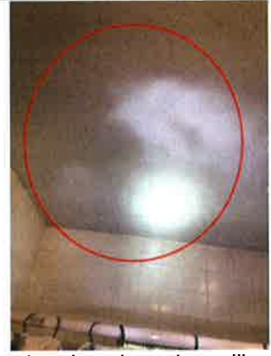
Discoloration along the ceiling.
