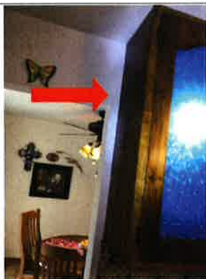
Crack along the wall.
