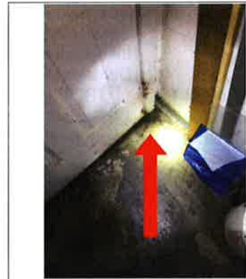
Moisture/dampness. An active or intermittent water source can cause mold growth.
