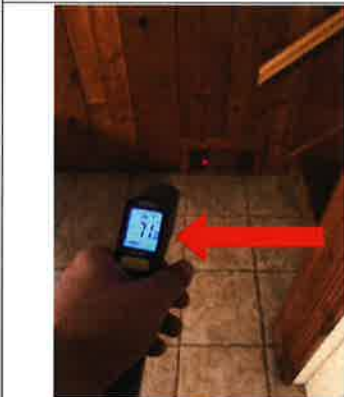
The photo identifies the temperature of the return air while the air conditioner was in operation. The approximate temperature of the return air was 71 degrees Fahrenheit.
