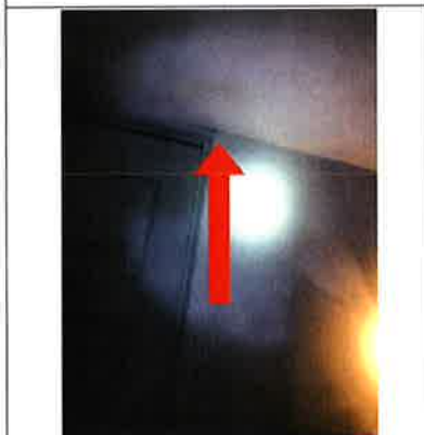
Slight cracking along the ceiling.
