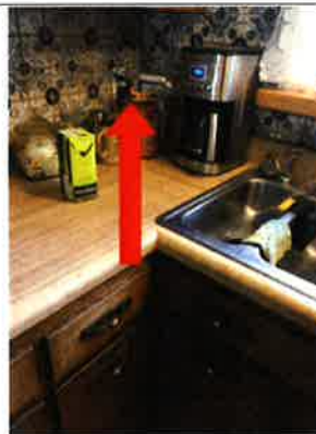
The receptacle is non GFCI protected.
