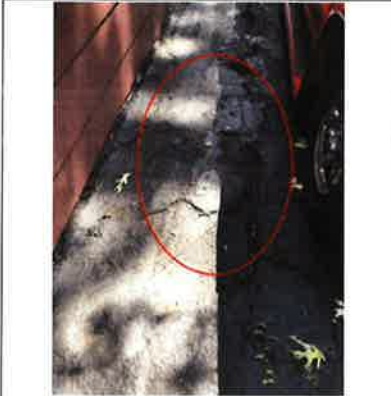
Deterioration along the driveway and uneven surfaces.
