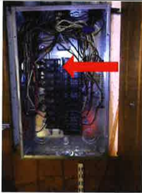
Main circuit breaker.
