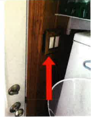
The switch is not flush with the wall thus creating a gap. This is a potential safety hazard.
