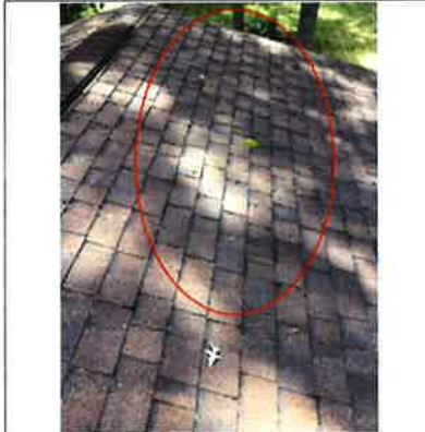
Biological growth along the roof. Biological growth has the potential to hold water. Asphalt shingles are not designed to hold water, they are designed to shed water.
