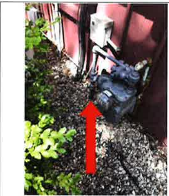
Main fuel shut off valve.
