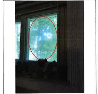
Insulated glass seal failure.
