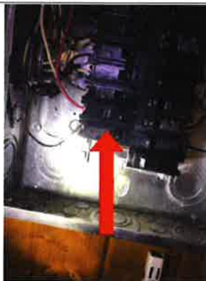
Oversized circuit breaker. A 40 amp circuit breaker should not have a wire that is smaller than an 8 gauge.
