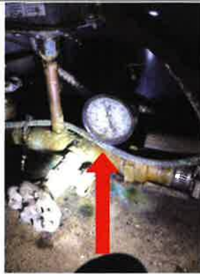
The well pressure was approximately 40 PSI and stayed consistent during the inspection.
