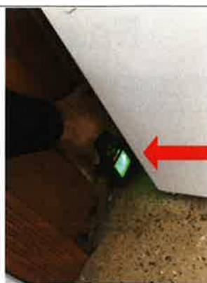
Moisture and discoloration observed along the base of the wall. An active or intermittent water source can cause mold growth.
