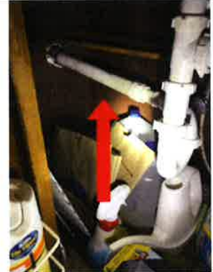
The drain/waste pipe is sloped the wrong way. This can potentially create slow drainage and/or blockage.
