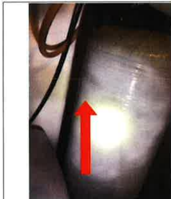
Condensation along the water softener. An active or intermittent water source can cause mold growth.
