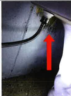
Mold like substance along the foundation wall. This is located behind the toilet in the basement.
