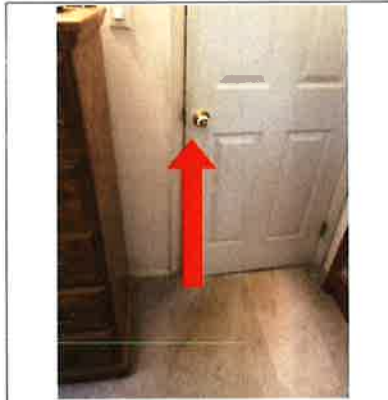
The door does not properly latch and the door drags the carpet.
