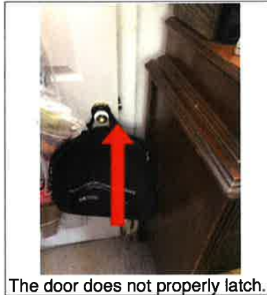
The door does not properly latch.
