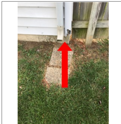
Damage along the siding.
