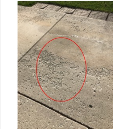
Deterioration/pitting along the driveway.
