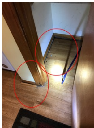
Signs of previous water damage along the walls and baseboards. This is adjacent to the dishwasher. An active or intermittent water source can cause mold growth.
