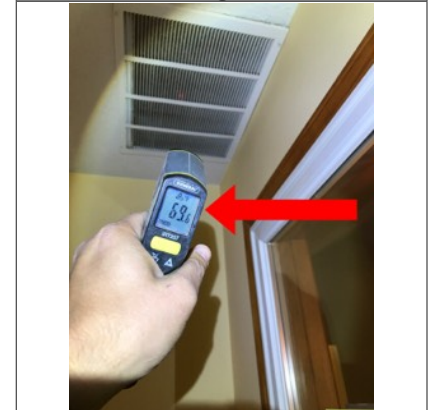
The photo identifies the temperature of the return air while the furnace was in operation. The approximate temperature of the return air was 69 degrees Fahrenheit.
