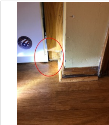
Standing water under the dishwasher. An active or intermittent water source can cause mold growth.
