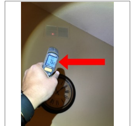
The photo identifies the temperature of the return air while the furnace was in operation. The approximate temperature of the return air was 75 degrees Fahrenheit.
