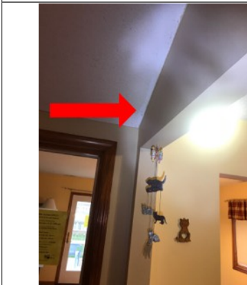
Discoloration along the ceiling.
