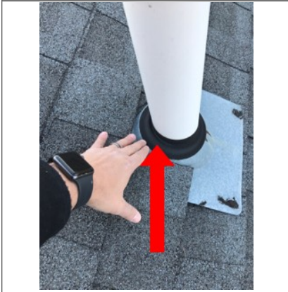
The rubber flashing around the plumbing vent is concave. This acts as a trap for water and snow, thus creating a potential leak point. Flashing is not designed to hold water, flashing is designed to shed water.
