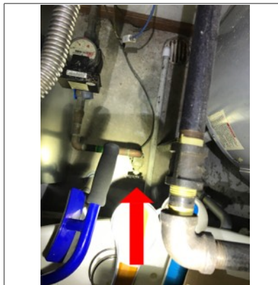
Main water shut off valve.
