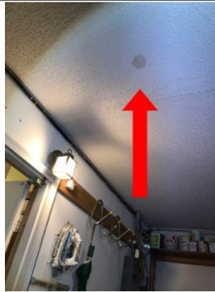
Discoloration along the ceiling.
