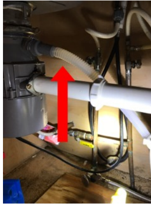
The dishwasher drain line does not have a high loop. A high loop helps prevent drain/waste water from flowing into the dishwasher and contaminating the clean dishes.
