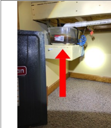
The condensation pump is unconventionally sitting in a plastic tub. The tub is filled with water. This is considered amateur craftsmanship and is a potential leak point.
