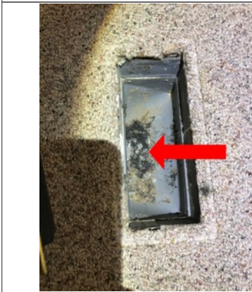
The HVAC ductwork is dirty.
