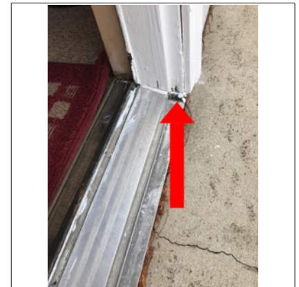
Rotted wood along the rear entry door.
