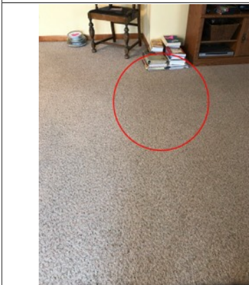
The floor slopes.
