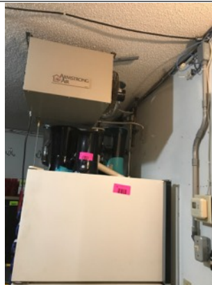
The garage furnace is inoperable. The display on the thermostat was blank (See photo 1A).
