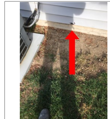
Damage along the siding.
