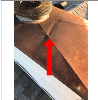
Dents/damage along the top plate.
