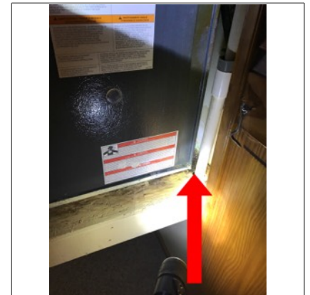
Signs of previous water damage along the condensation line. An active or intermittent water source can cause mold growth.
