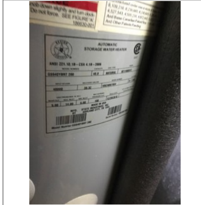
Water heater data plate.
