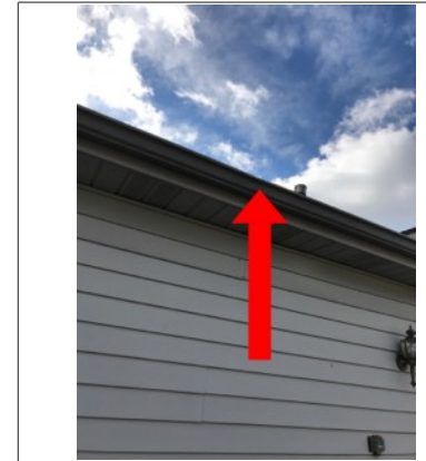
Dents along the gutter system.
