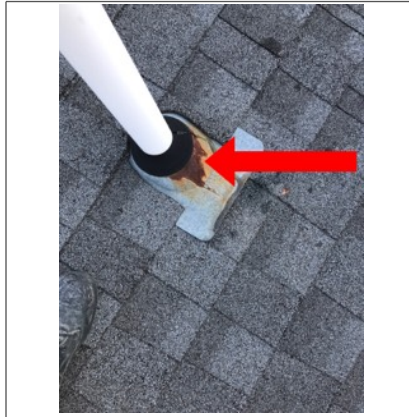
Rust/corrosion along the flashing. This is a potential leak point.
