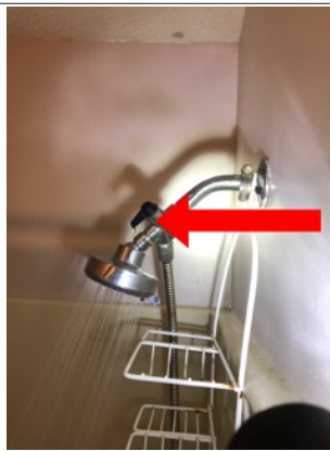
The showerhead leaks during operation.
