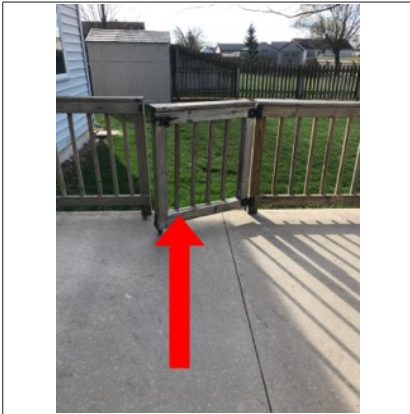
The gates are difficult to operate.
