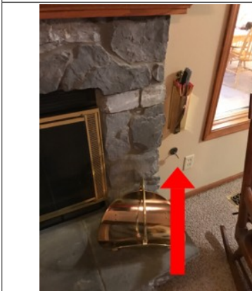
The fireplace is gas. However, there is not an apparent electronic ignition to the fireplace, it is beyond the scope of a general home inspection to light gas fireplaces that do not have an electronic ignition.
