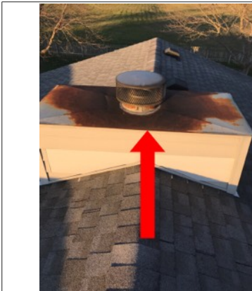
Rust/corrosion along the top plate. The rust/corrosion is a potential leak point.
