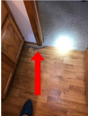
Discoloration along the floor.
