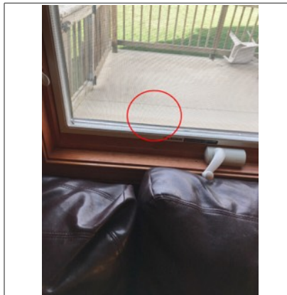
Small holes along the screen.
