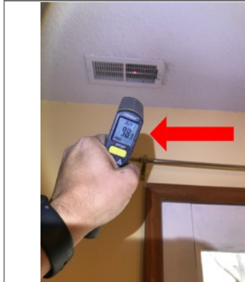
The photo identifies the temperature of the supply air while the furnace was in operation. The approximate temperature of the supply air was 98 degrees Fahrenheit.
