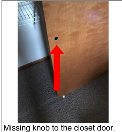
Missing knob to the closet door.
