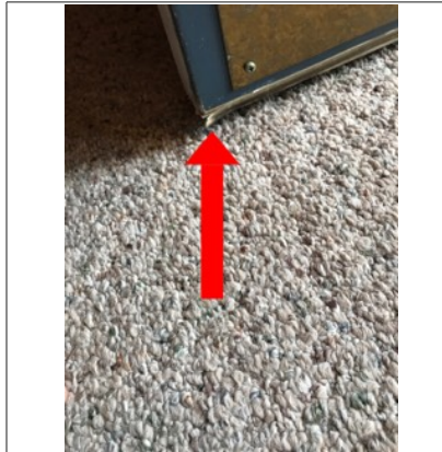
Torn weatherstrip along the main entry door.
