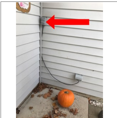
The receptacle has an open neutral. Also, the exterior wiring is unconventional. The receptacle identified by the arrow is mounted to the exterior wall and is plugged into the receptacle below it. This is considered amateur craftsmanship.
