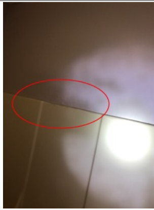
Signs of previous repairs along the wall. This is located above the shower wall.
