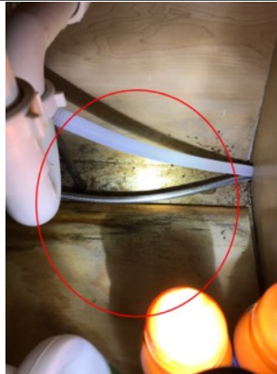
Moisture observed underneath the sink and signs of previous water damage. An active or intermittent water source can cause mold growth.
