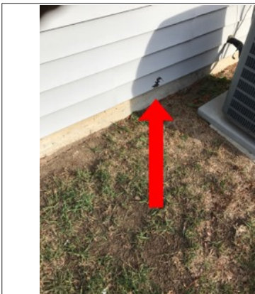
Damage along the siding.
