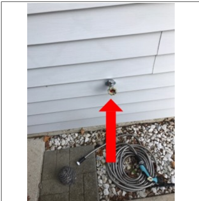
The hose bib is loose. The hose bib is inoperable.
