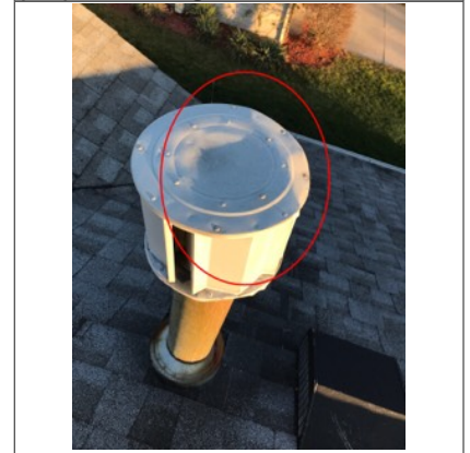
Dents along the flue.
