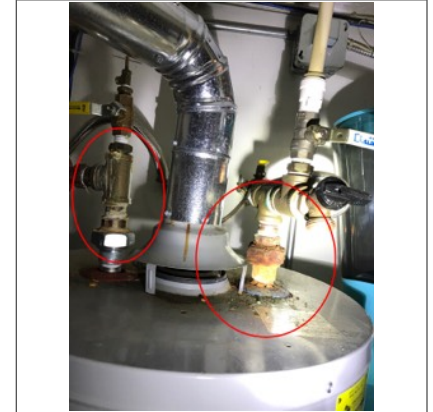
Rust/corrosion along the water supply lines. This is located above the water heater.
