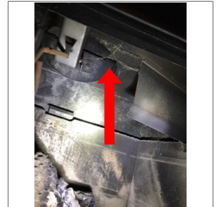
Spider webs within the fireplace. This is an indication that the fireplace has not been regularly used for an extended period of time.
