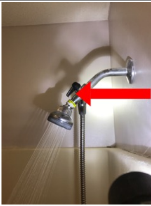
The showerhead leaks during operation.
