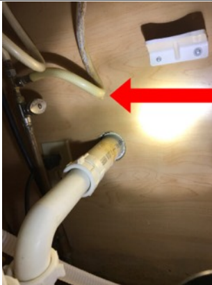
Active leak underneath the sink.
