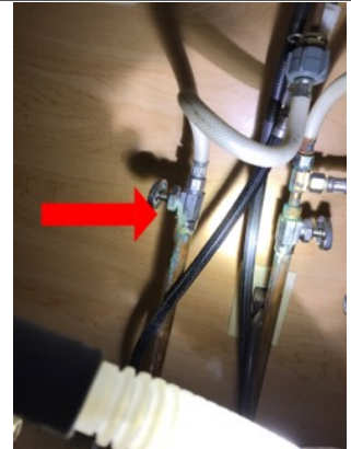
Corrosion along the water supply lines. This is located underneath the sink.
