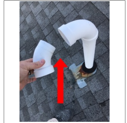
The fitting along the plumbing vent is not glued. Ideally, the arched fittings on the vent are considered abnormal. Vertical termination is recommended for proper venting.
