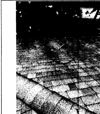
Tree branches/debris along the roof. Falling tree branches can damage the roof shingles.
