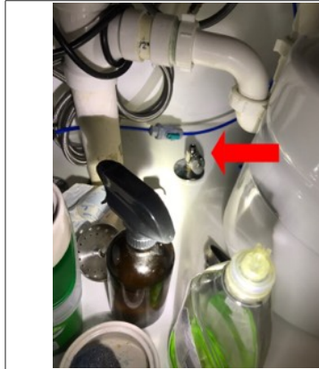
Uncapped water line.
