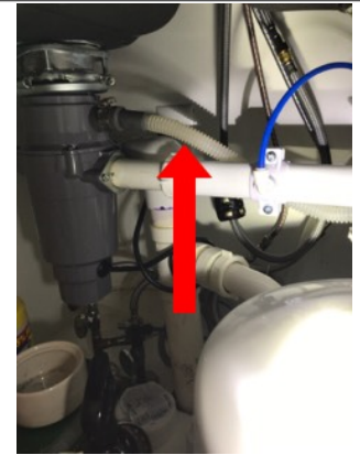
The dishwasher drain line does not have a high loop. A high loop helps prevent drain/waste water from flowing into the dishwasher and contaminating the clean dishes.
