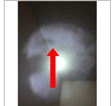
Apparent nail pop along the ceiling.
