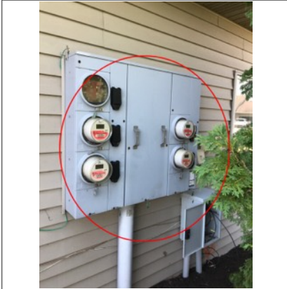
One of the disconnect switches is the main for the house.
