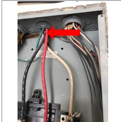
Loose/unused wire. No voltage detected. Ideally, unused wires should be removed.
