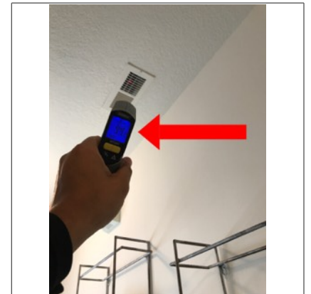
The photo identifies the temperature of the supply air while the furnace was in operation. The approximate temperature of the supply air was 94 degrees Fahrenheit.
