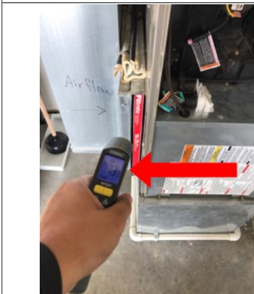
The photo identifies the temperature of the return air while the furnace was in operation. The approximate temperature of the return air was 73 degrees Fahrenheit.
