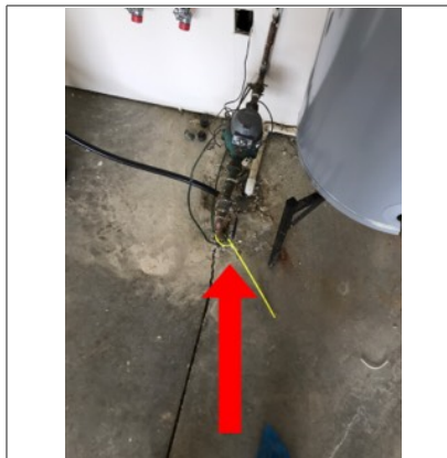
Main water shut off valve.
