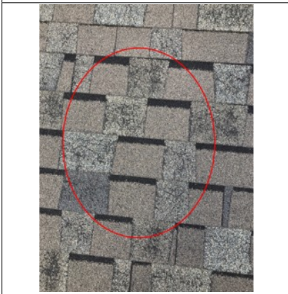
Cracks and granule loss along the roof.
