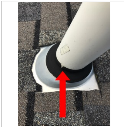
Deterioration along the flashing around the plumbing vent. This is a potential leak point.
