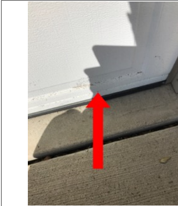
Flaking/peeling along the overhead garage door.
