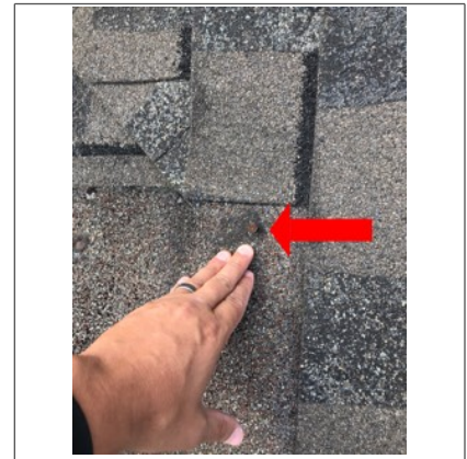
Exposed nailheads along the roof. Exposed nailheads are potential leak points.
