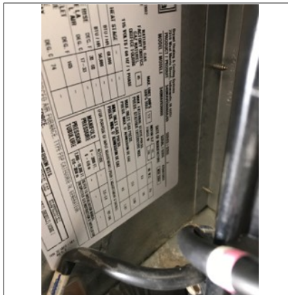
Furnace data plate.
