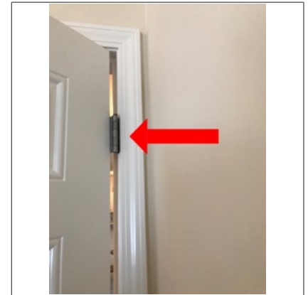
The door hinge is loose making the door out of alignment.
