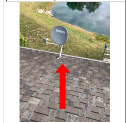
Dish mounted to the roof. While mounting a dish to a roof is a common practice, it is not a recommended practice due to the anchor bolts that penetrate the roof shingles, underlayment and sheathing thus creating a potential leak point.
