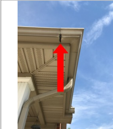
Signs of previous repairs along the gutter. Some of the seams have an adhesive/caulk applied to them. This is an indication that the gutter system leaked at some point in the past.
