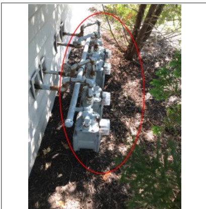
One of the fuel shut off valves is the main for the house.
