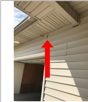
Gap along the siding.
